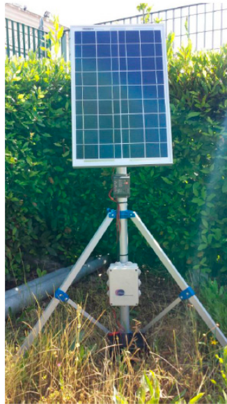
Figure 29. One of the nodes (enclosed in the white box) with its solar panel.
