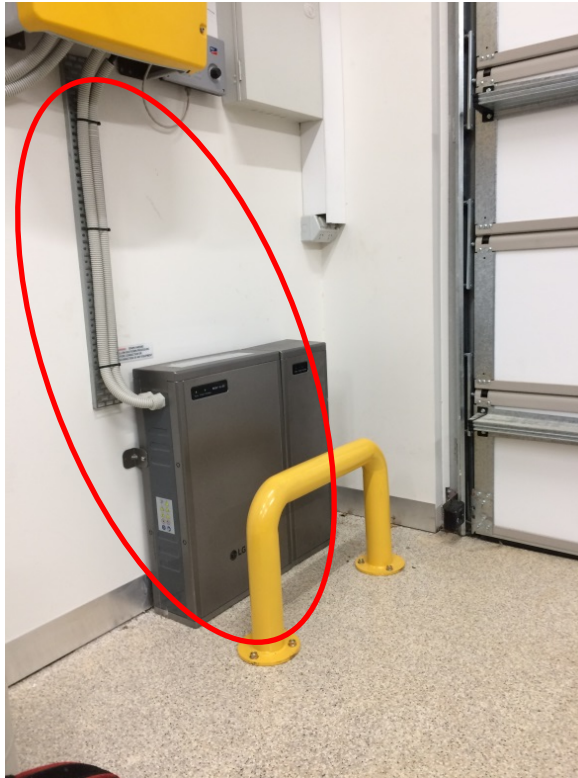
Figure 1 Scope of these guidelines: The battery system including cabling up to PCE terminals
