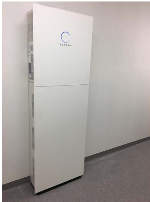
Figure 4 Scope of these guidelines: Installation of pre-assembled integrated battery energy storage systems (pre-assembled BESS)
