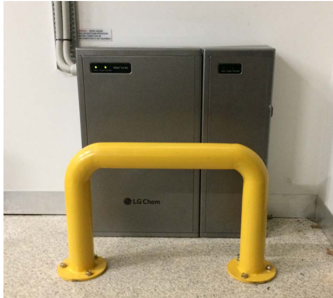
Figure 11 Battery system mechanically protected by a bollard in a garage
