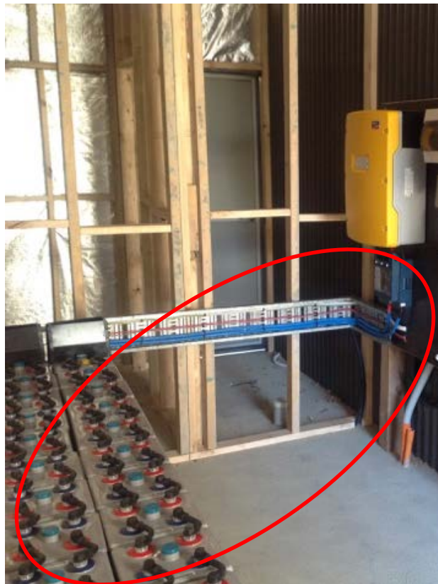
Figure 2 Scope of these guidelines: Installation of pre-assembled integrated battery energy storage systems (pre-assembled BESS)
