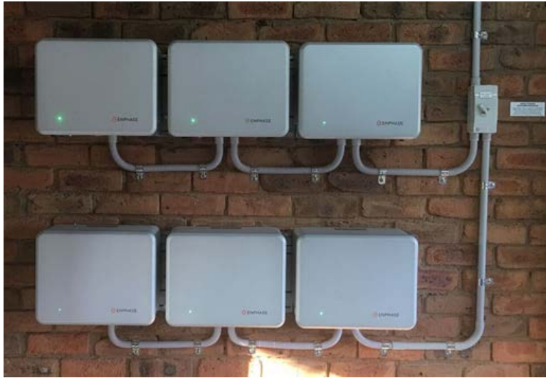
Figure 3 Scope of these guidelines: Installation of pre-assembled integrated battery energy storage systems (pre-assembled BESS)
