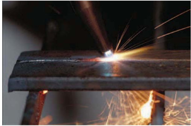
FIGURE 21-82 The torch is rotated to allow the preheating of the plate ahead of the cut. This speeds the cutting and provides better visibility of the line being cut. Larry Jeffus
