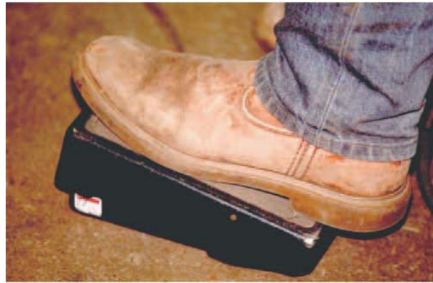
FIGURE 16-16 A foot-operated device can be used to increase the current. Larry Jeffus
