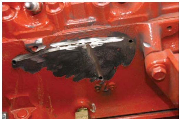
FIGURE 5-7C Grind a U-groove all the way along the crack. (continued) Larry Jeffus
