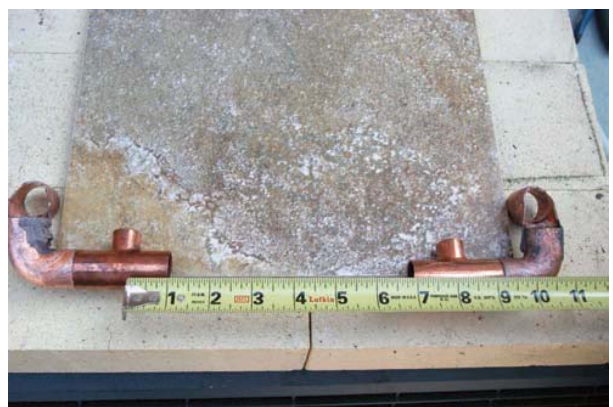
FIGURE 20-56 Lay the pipe on the tile to check the length of the copper pipe. Larry Jeffus
