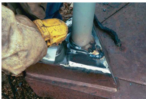
FIGURE 1-8 Angle grinding a weld to prepare it for finish painting. Larry Jeffus
