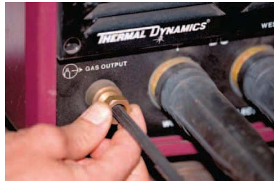
FIGURE 15-36 Tighten each fitting as it is connected to avoid missing a connection. Larry Jeffus
