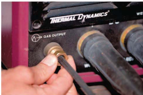
FIGURE 16-7 Tighten each fitting as it is connected to avoid missing a connection. Larry Jeffus
