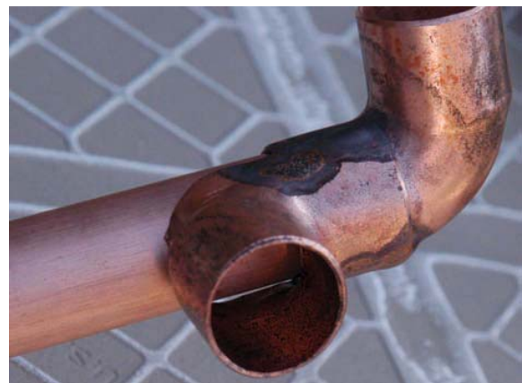
FIGURE 20-64A The inside of the fitting will have a heavy oxide. Larry Jeffus
