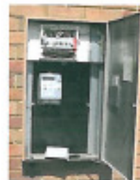
Main Switchboard/Metering Enclosure
