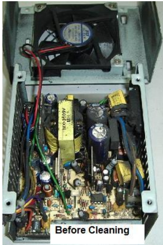
Figure 20.6- Dirt Inside The Power Supply
