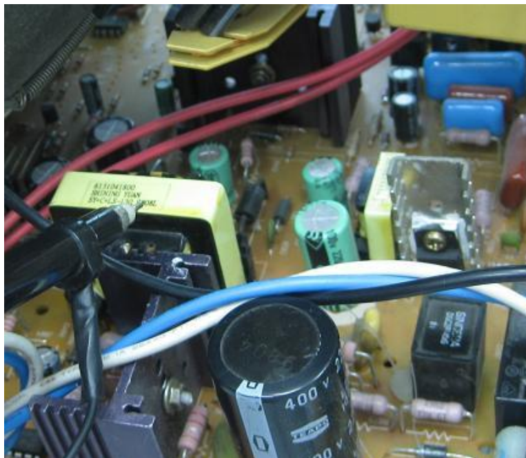
Figure 12.17- Placing The Scope Probe On Switch Mode Transformer
