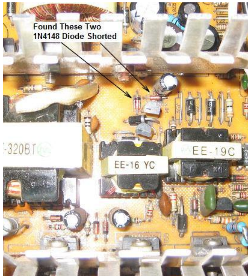
Figure 20.11- Low Output Voltages Could Be Caused By Shorted Signal Diodes In The Secondary Side
