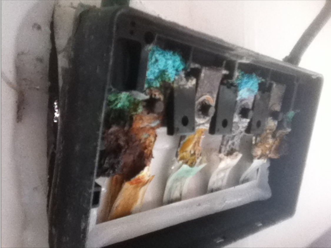
Figure 19. Manual inspection and testing requires opening NEMA-rated enclosures. The integrity of any enclosure seal must be restored after opening to avoid moisture damage as in this module junction box. Photo by Andy Walker, NREL
