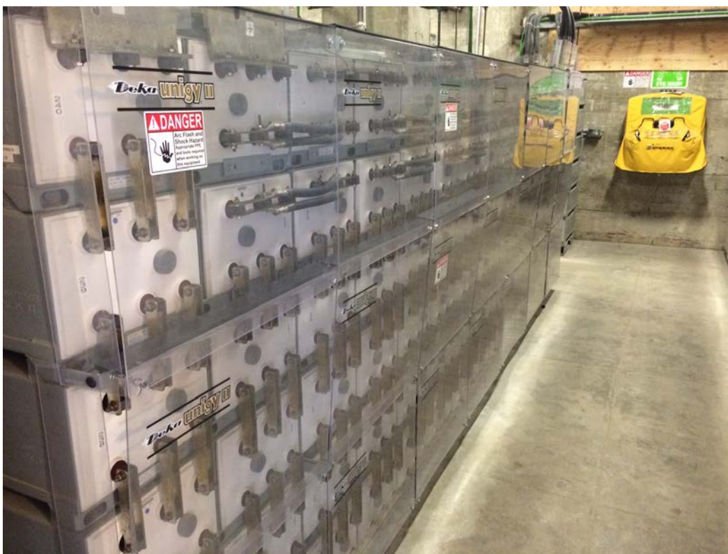
Figure 13. The National Park Service budgets, ideally, $100,000 per year for O&M of this PV energy storage system (308 kW PV; 1,920 kWh battery) on Alcatraz Island. Photo by Andy Walker, NREL
