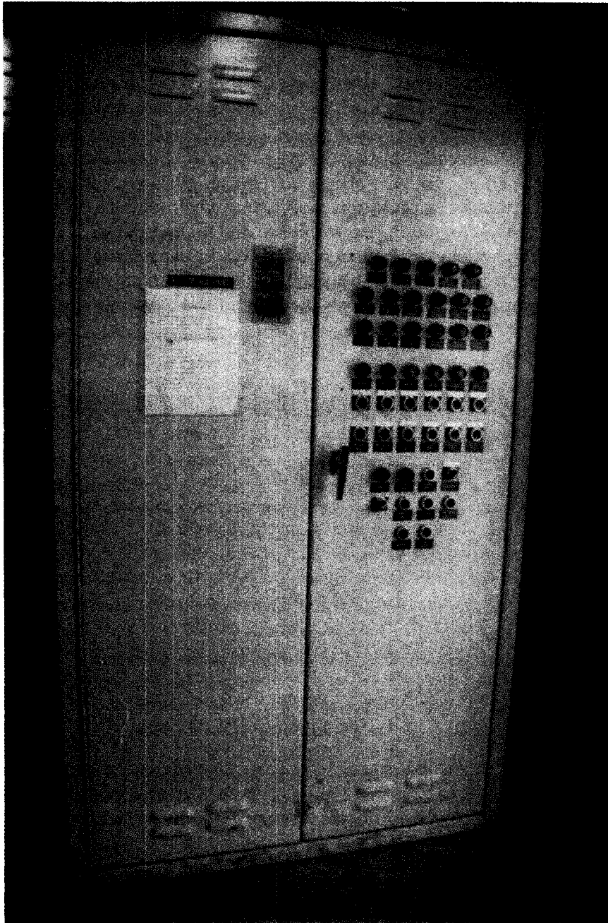
Figure 10-8. Front View of RTU Marshaling Panel (Courtesy: Imperial Oil Resources, Ltd.)
