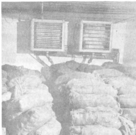
Figure 15.—Blower-type cooling units in a refrigerated room. (Photo courtesy of Blount Seafood Corporation)
