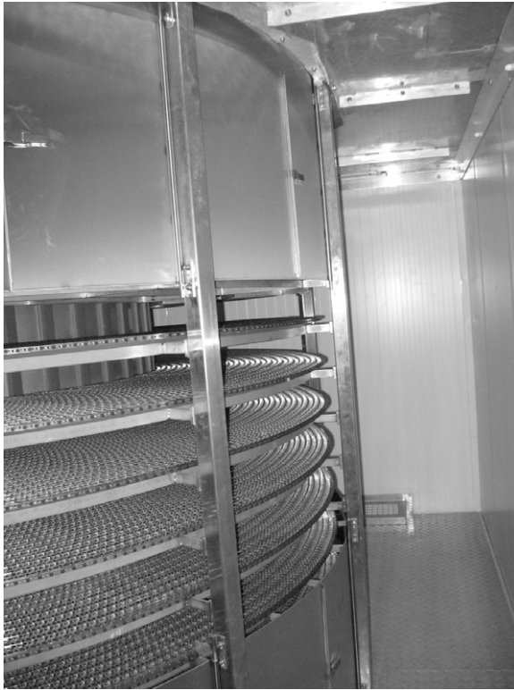
Figure 14.2 View of spiral freezer (Star Refrigeration)
