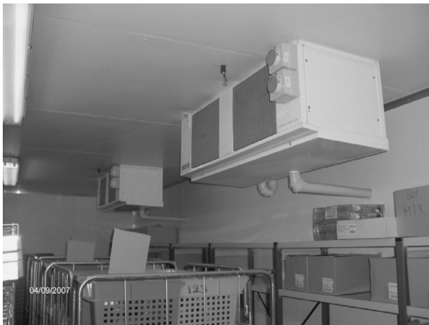
Figure 15.8 Ceiling-mounted coolers (Michael Boast)
