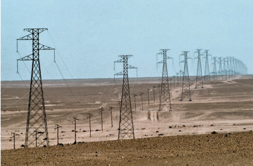
High-voltage power lines carry electricity for miles across the Namibian Desert in Africa.
