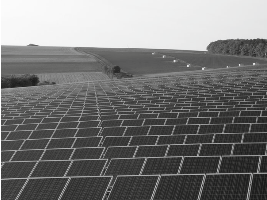
Fig. 4.9. Ground-based photovoltaic plant [10]
