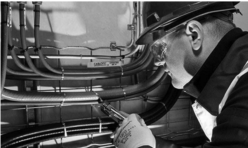
Figure 5.8 High-quality offshore wiring and cabling [Source: Cablofil]
