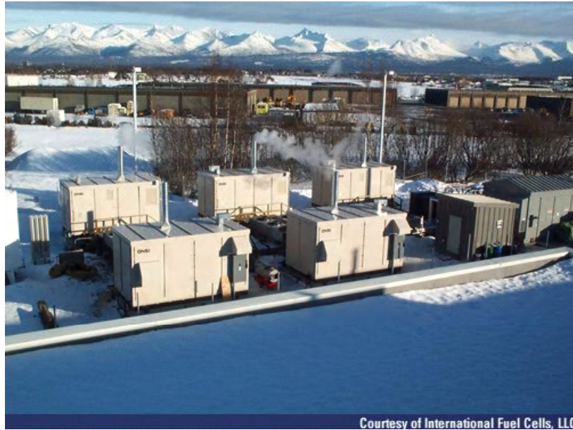
Figure 5.41. International fuel cells. Installation of five PC25 units of 200 kW at the Regional USPS Mail Sorting Center at Anchorage, Alaska
