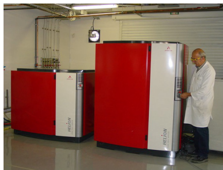
Figure 5.44. Hélicon stationary generator for 20 kW auxiliary supply (2005) (source: CEA)
