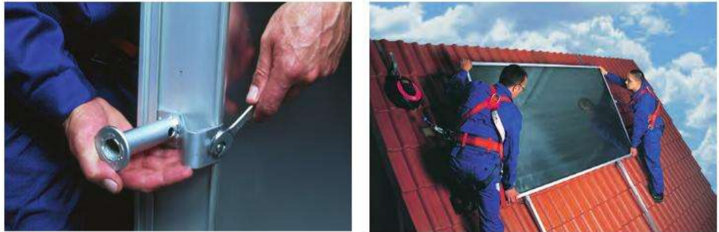
Figure 4.22. Example of on-roof installation with flat plate collectors Source: Wagner and Co., Cölbe
