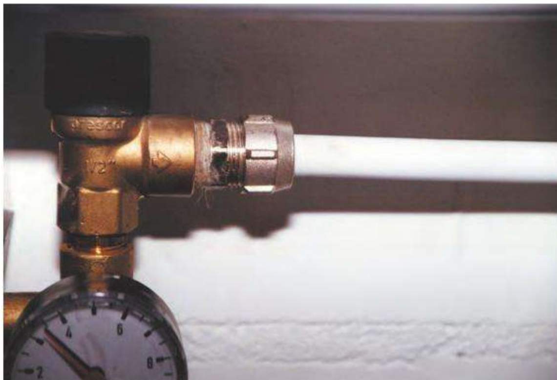
Figure 4.54 Incorrect PE pipe as exhaust line
