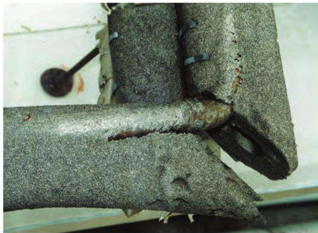
Figure 4.53 Damaged thermal insulation
