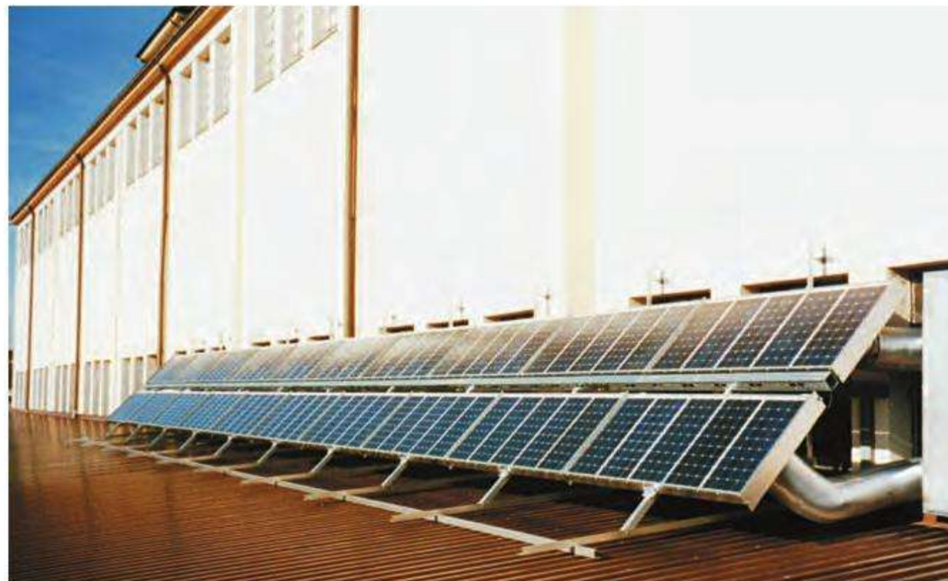
Figure 8.7. Hybrid collectors for solar air heating and generation of electricity for an automotive paint shop (Manufacturer: Grammer Solar+Bau GmbH, Amberg)
