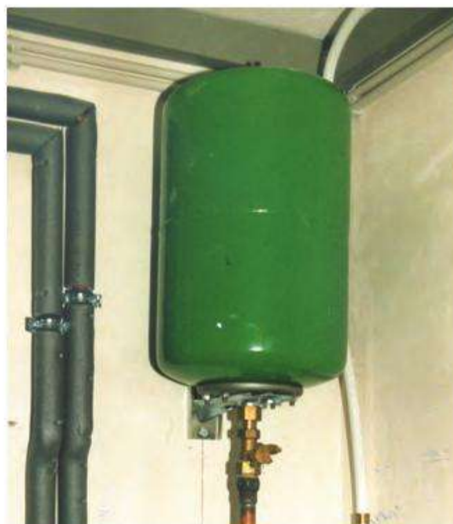
Figure 4.57 False expansion vessel connection from below
