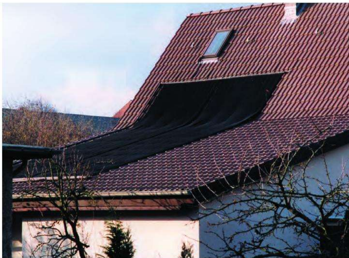
Figure 7.24. Private solar system for pool heating
