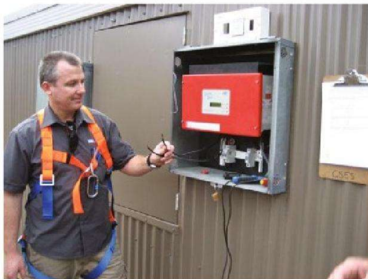
Figure 5.3 An electrician tests a grid-interactive inverter
