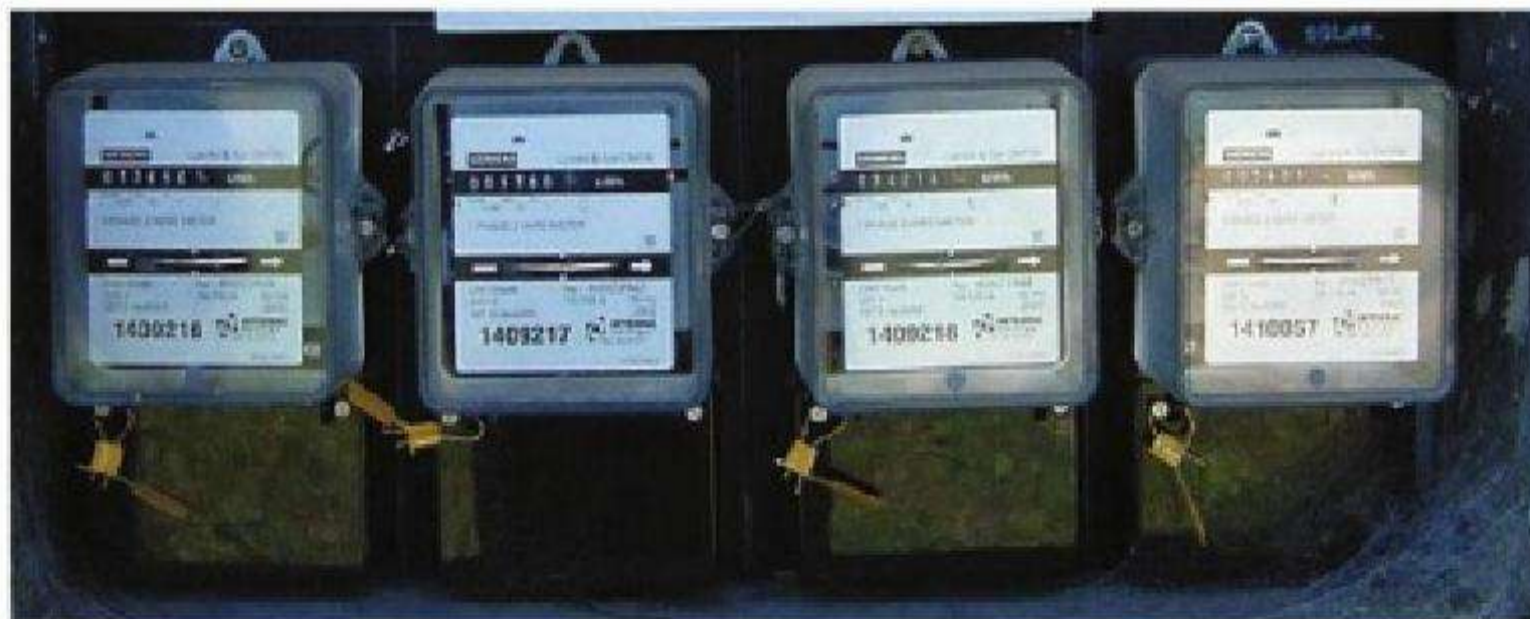
Figure 5.42 Multiple meters are common, often for off and on peak demand metering and large appliances like ducted air-conditioning
