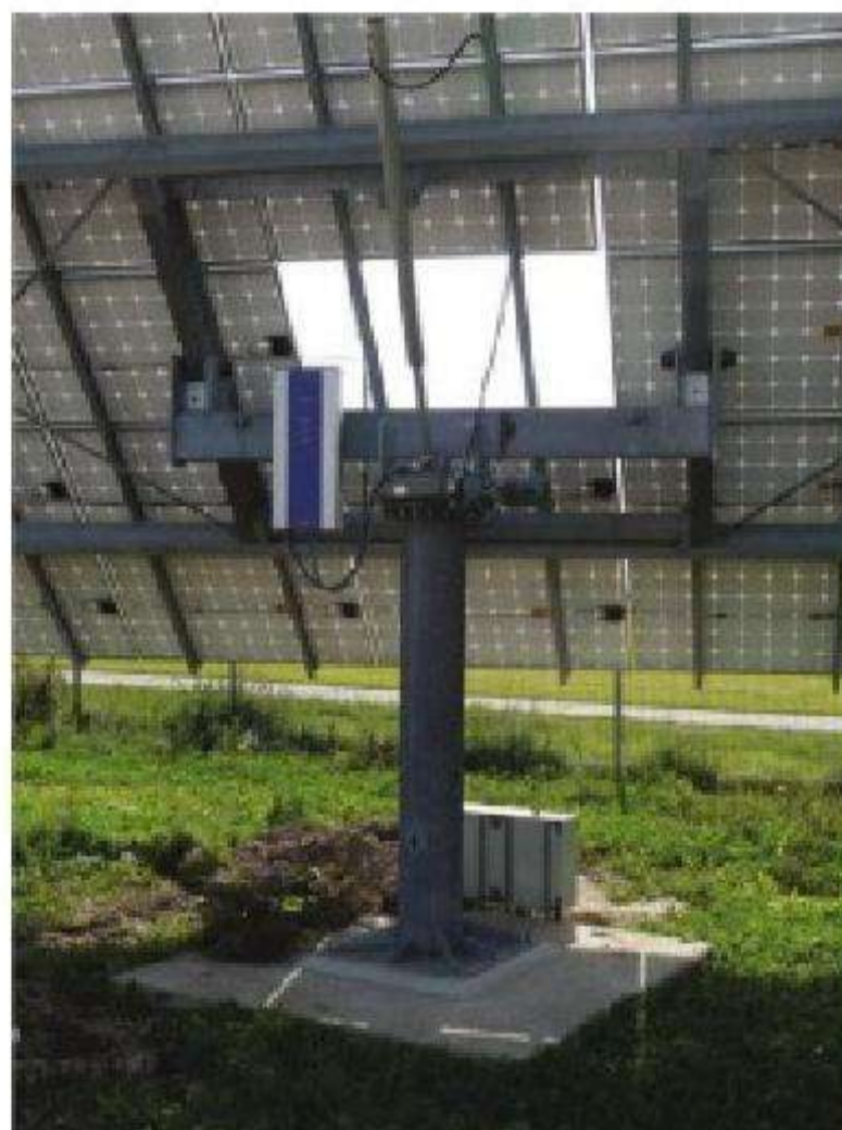
Figure 6.17 The tracking hardware can be seen on the back of this array
