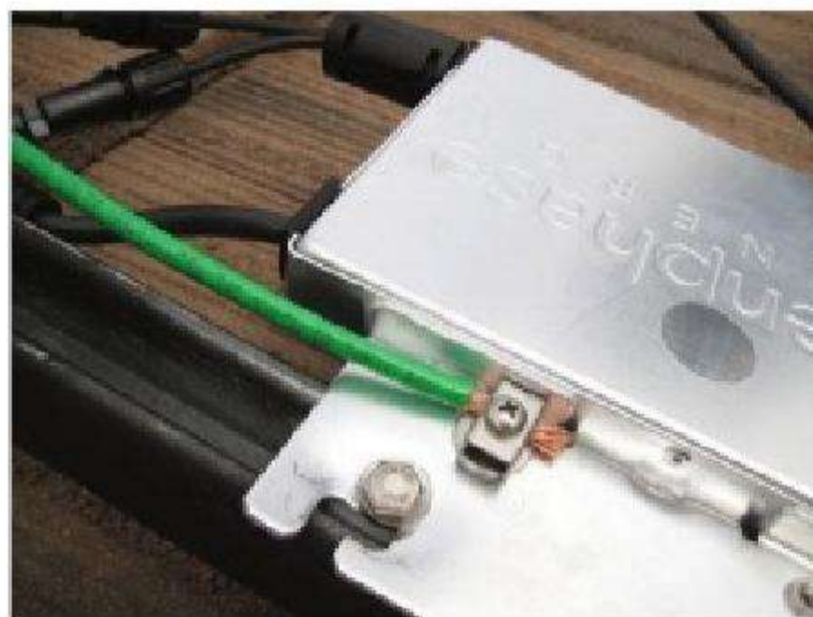
Figure 14.22 In accordance with the National Electric Code (NEC), all metallic parts of the PV array which could potentially become exposed to live current are mechanically bonded to the earth (grounded/earthed) using either bare copper or green cables. This includes the PV module frames, mounting system and conduit as well as the individual micro-inverters as shown above
