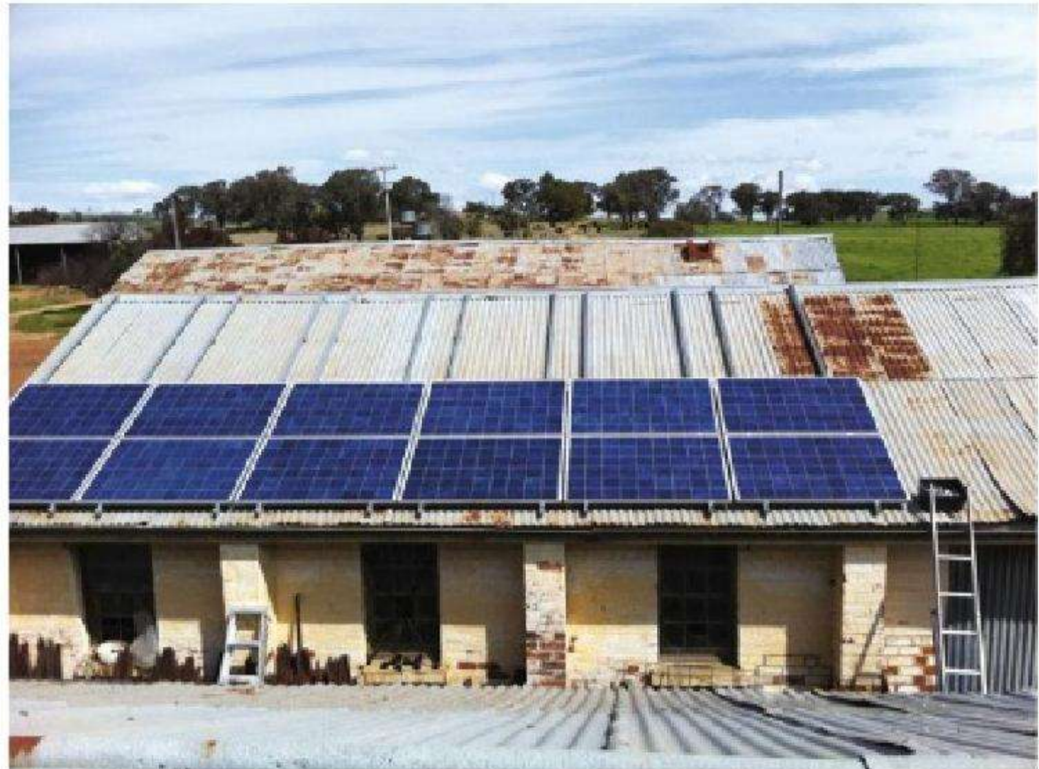
Figure 14.29 In this photograph the metal rails that make up the mounting structure are clearly visible
