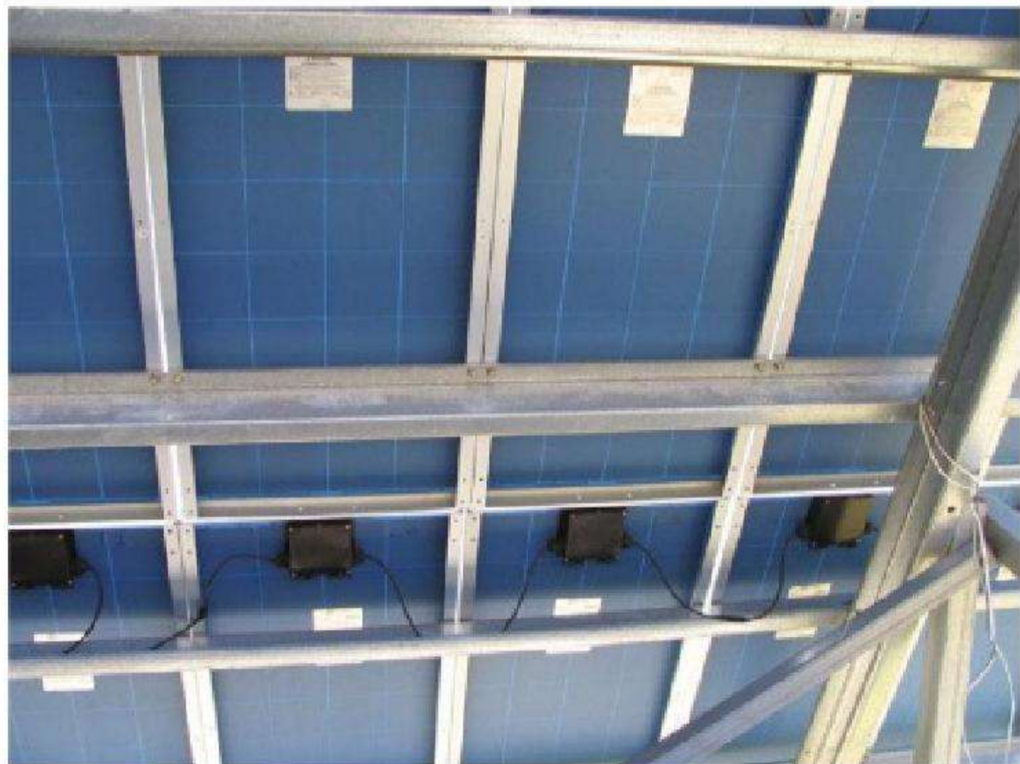
Figure 5.24 Module junction boxes on the back of modules in a PV array
