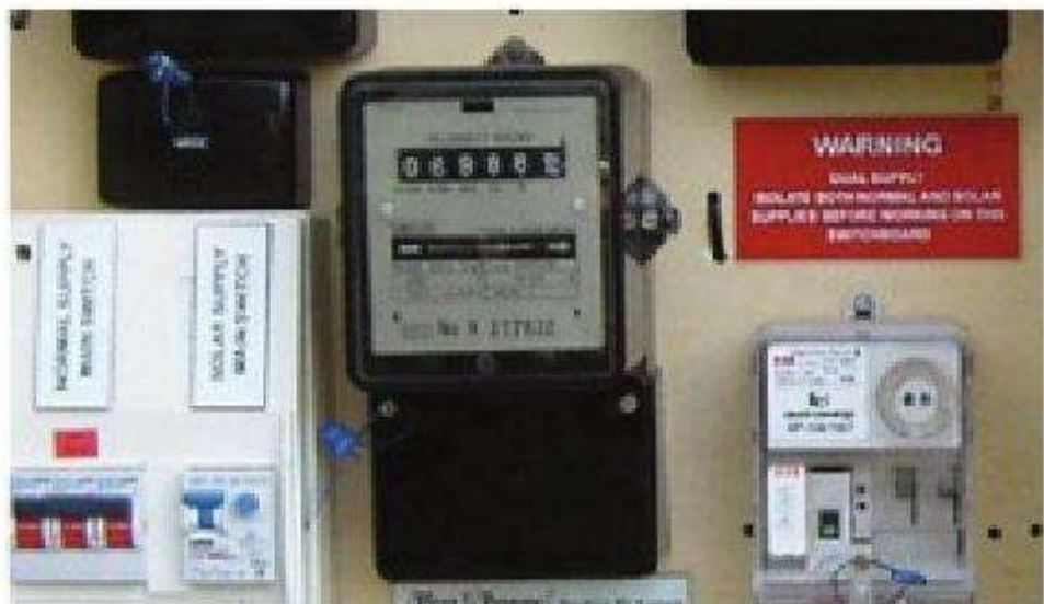
Figure 5.34 Rotating barrel style meter, here shown accompanied by signage for a PV installation
