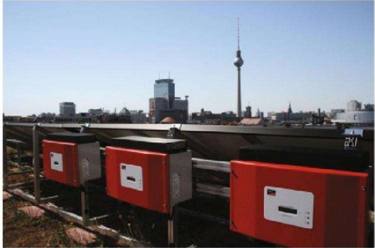
Figure 14.1 Three inverters are used, one for each array Source: Alberto Gallego
