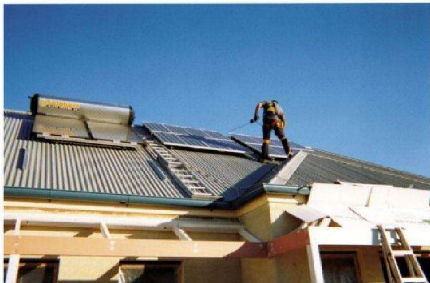
Figure 1.3 An electrician installing a solar system that includes both a solar hot water system (left) and a solar electric system (right)
