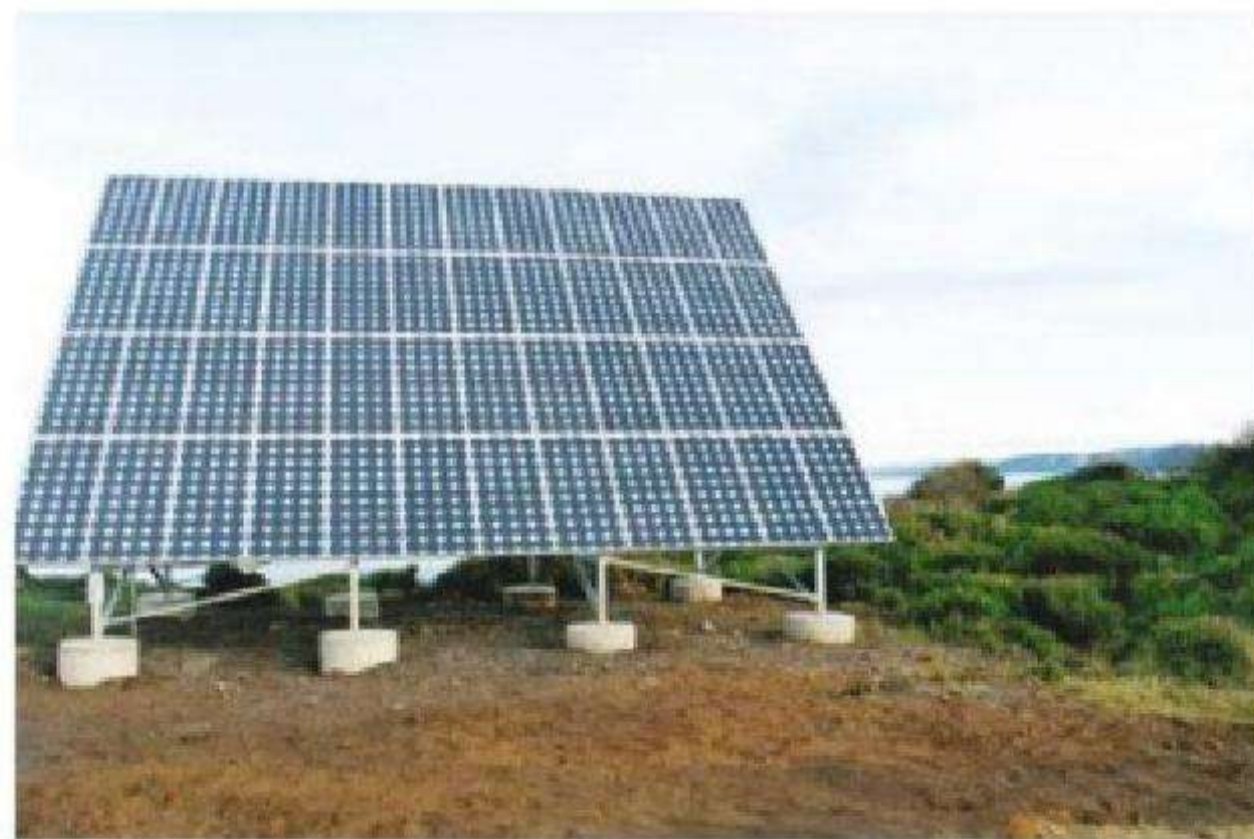
Figure 6.13 Large ground-rack mounted installation
