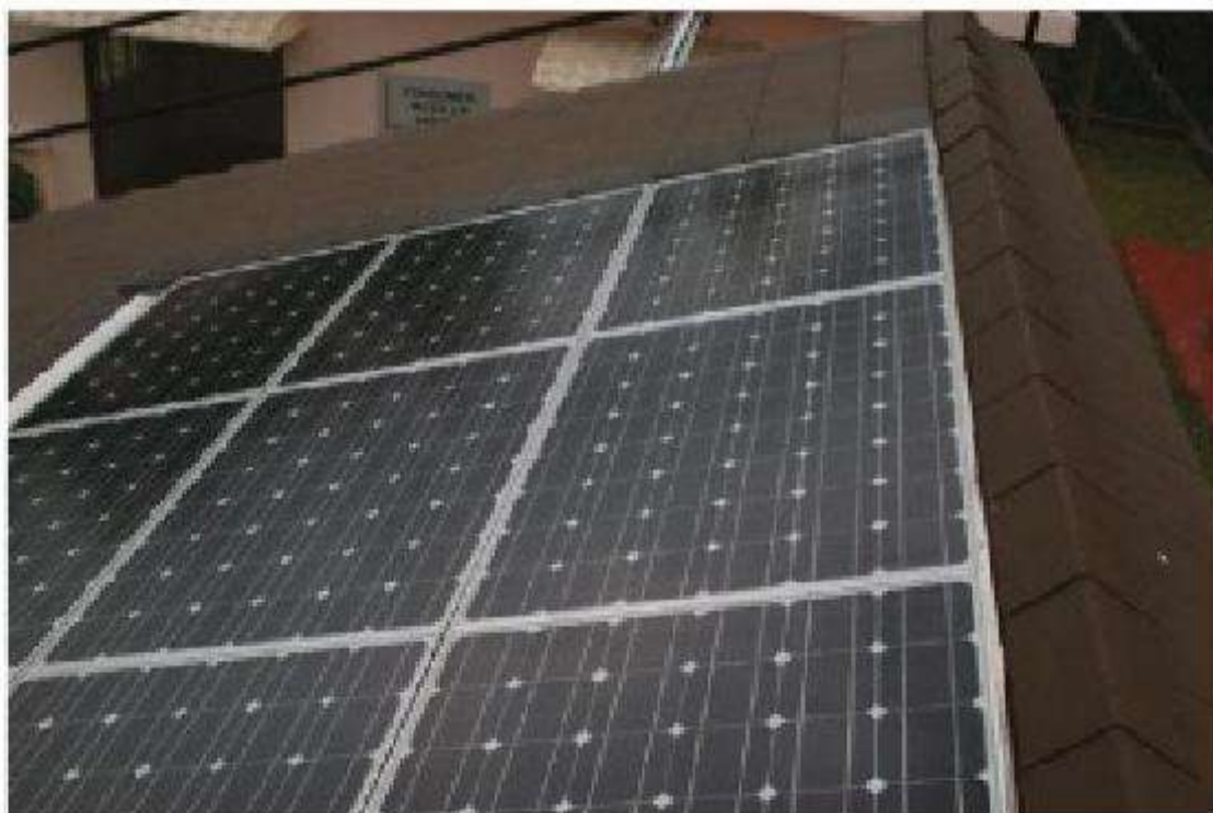
Figure 4.9 PV array composed of monocrystalline modules
