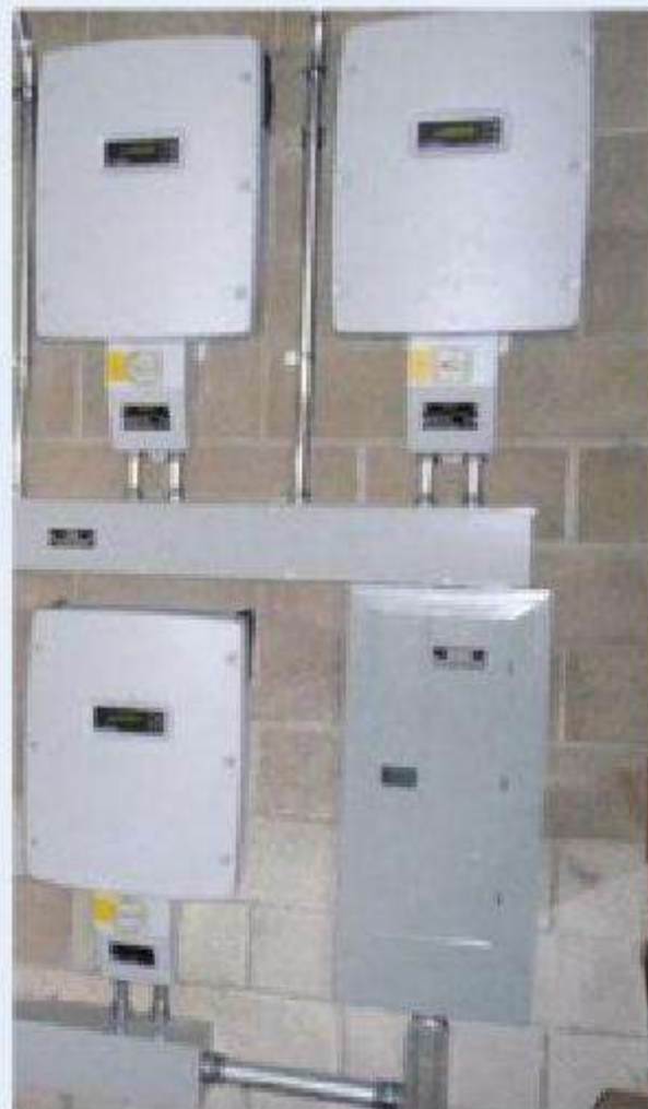
Figure 5.30 These inverters are designed for the US market and incorporate a large UEDS beneath the inverter
