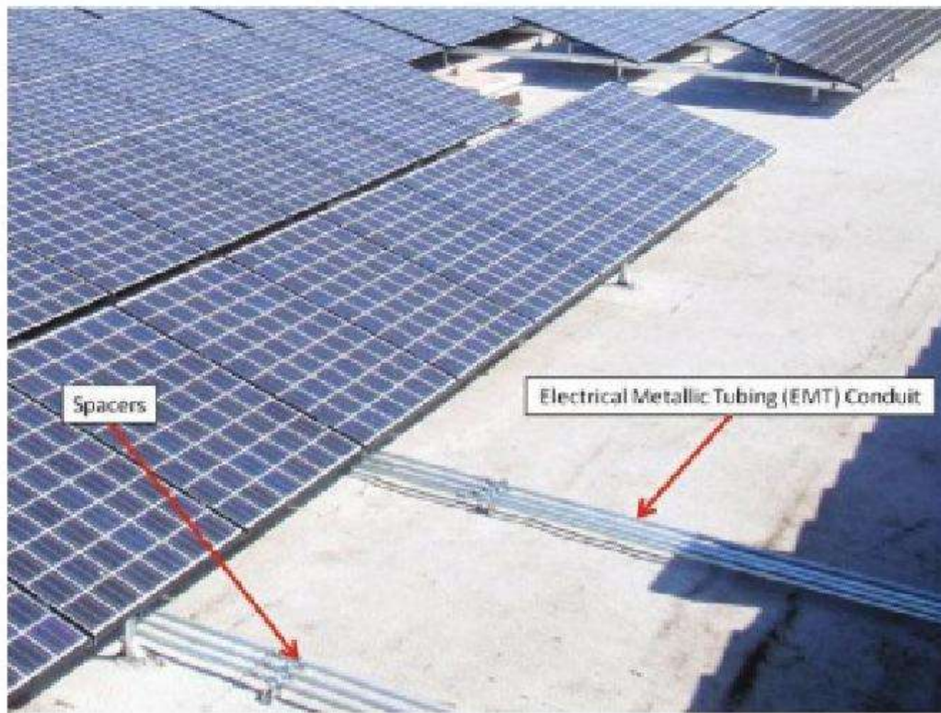
Figure 14.13 The DC conductors are housed inside a metallic conduit as per the guidelines in the National Electric Code (NEC). The 2008 NEC states that conduit in direct contact with a roof under full sunlight will experience an internal temperature of 33°C (60°F) above ambient while conduit that is mounted between 0.5 and 3.5 inches above the roof (as in this system) will experience an internal temperature of 22°C (40°F) above ambient. It is for this reason that the installers have mounted the conduit several inches above the surface of the roof
