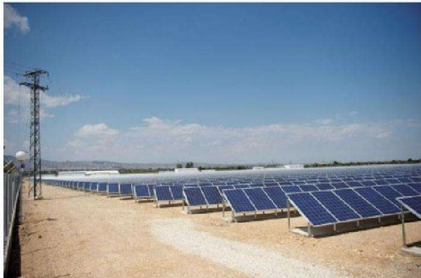
Figure 1.9 Alicante, Spain, 5.6MWp central PV system
