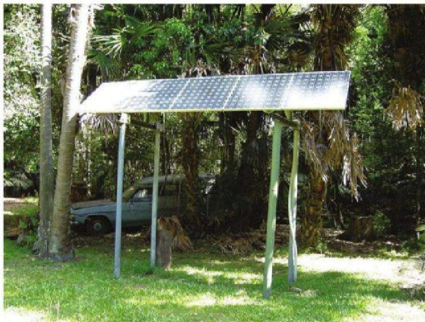
Figure 7.4 Poorly chosen site where trees are shading the PV array
