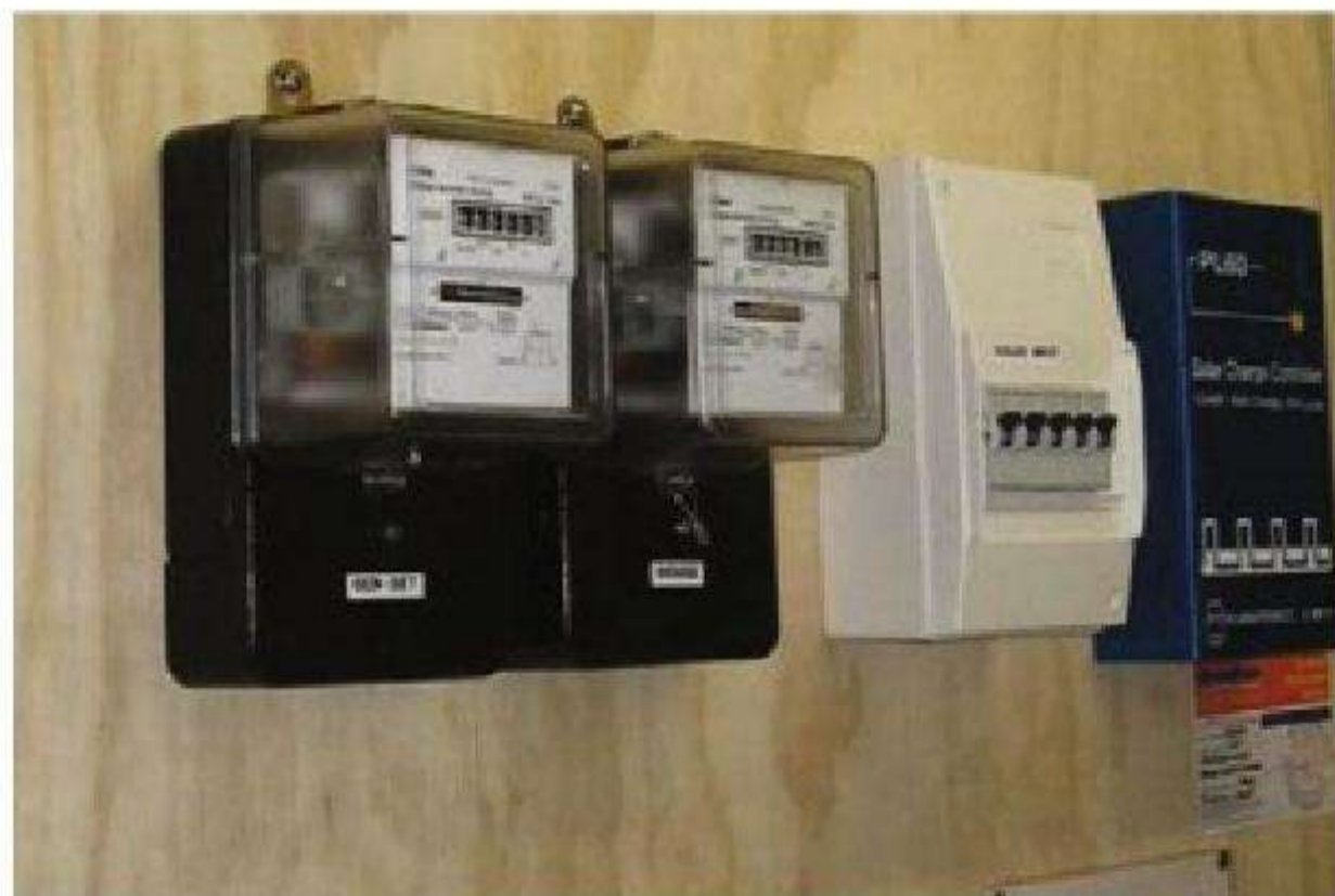
Figure 5.40 Two metering devices, one measuring the power generated and one measuring the power used
