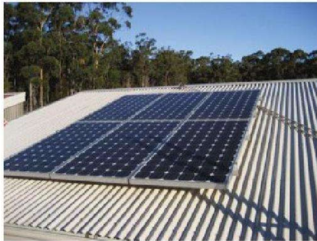
Figure 4.22 Even this small shadow can reduce the amount of electricity a module produces – a small shaded area can, under certain circumstances reduce module output by 80–90 per cent as well as affecting the rest of the array
