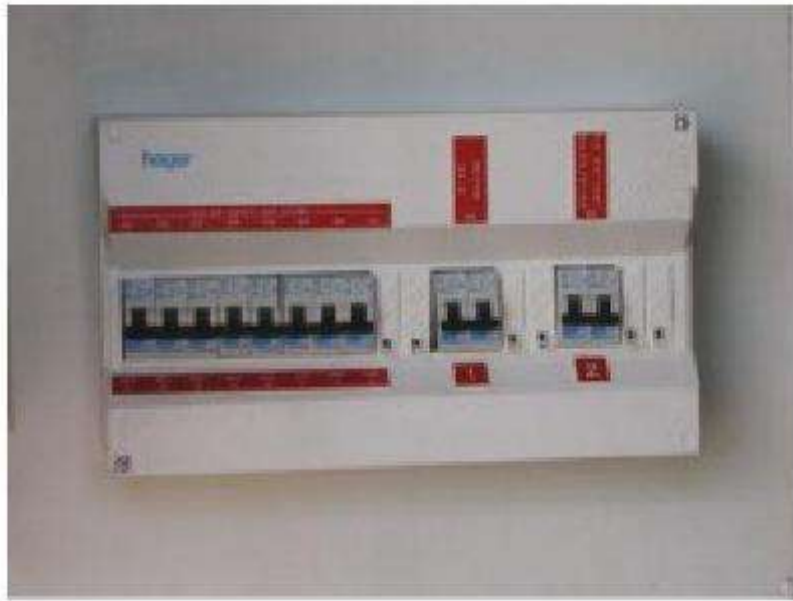
Figure 5.26 Circuit breakers in a grid-tied PV system
