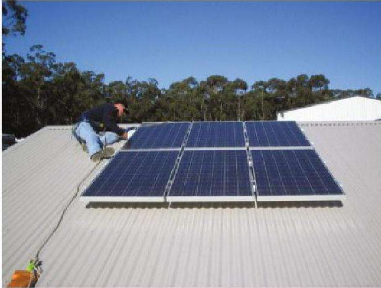
Figure 10.6 An electrician installs a small white PV combiner box next to the array
