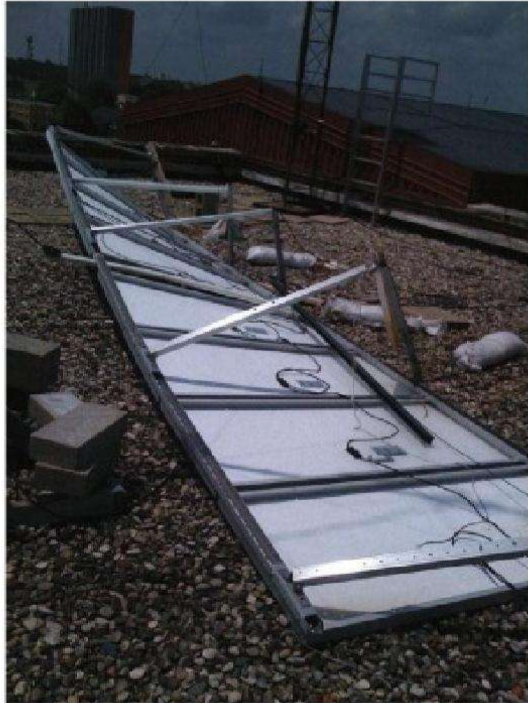
Figure 13.6 Severe winds can cause damage to poorly anchored arrays
