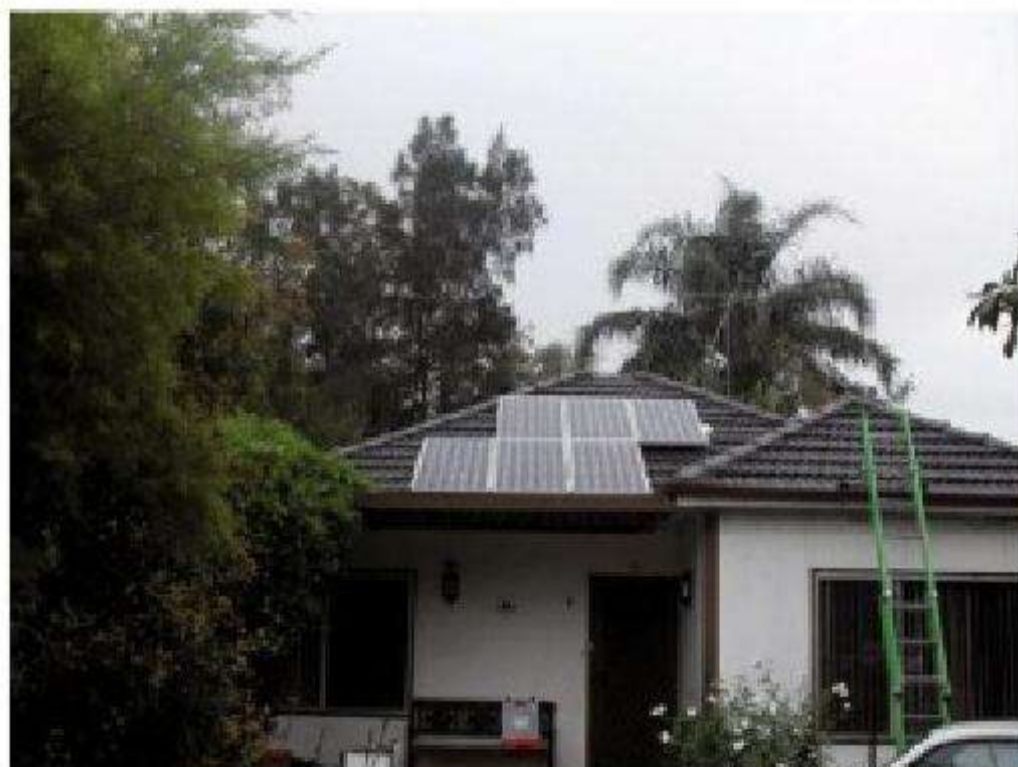
Figure 1.11 A residential PV system
