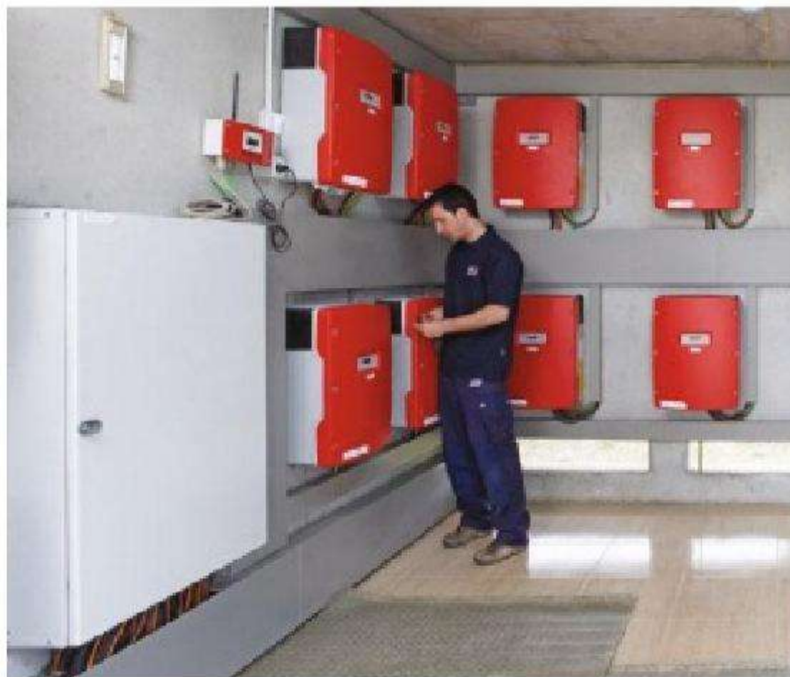
Figure 5.15 For very large installations a whole room of central inverters may be required. These are SMA Sunny Mini Central inverters
