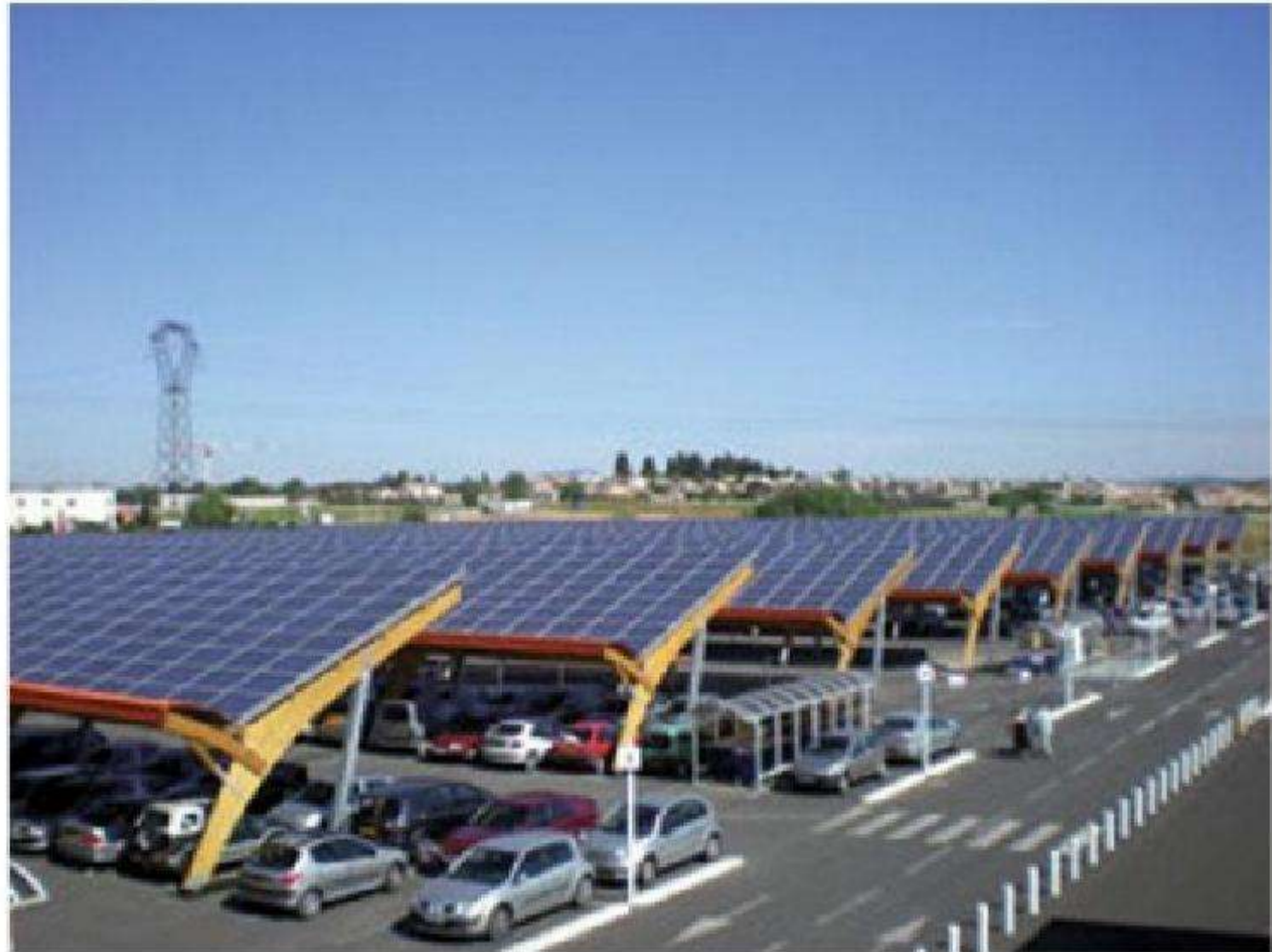
Figure 6.10 BIPV awnings developed by Sunvie and integrated into a car park; this 1.15MWp installation is located in St Aunès, France
