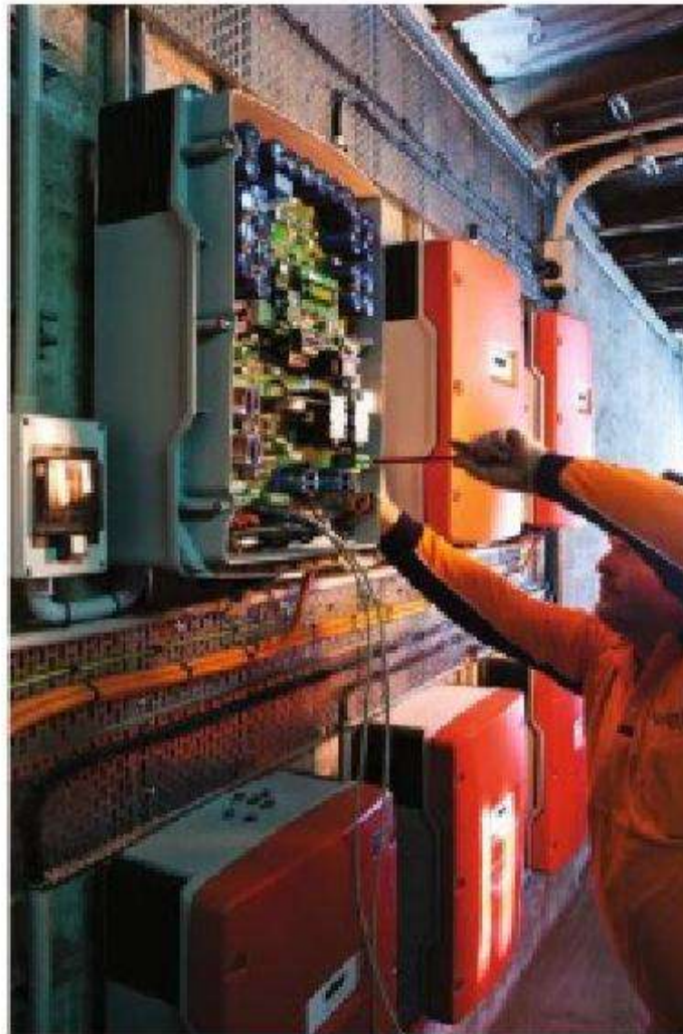
Figure 5.12 Multi-string inverters installed by Solgen Energy on Cockatoo Island for Sydney Harbour Federation Trust
