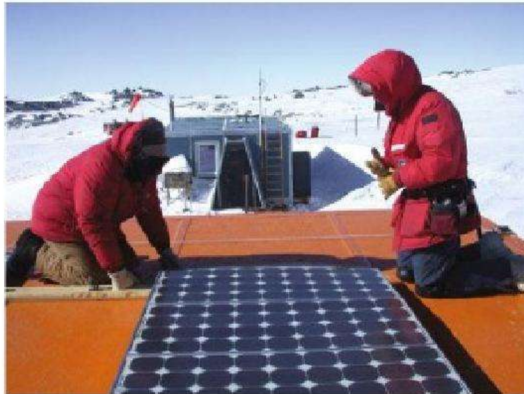
Figure 4.20 PV modules perform well in cold and sunny areas. They are often used as a power source in Antarctica during the summer. However, because there is so little light in winter, diesel generators are typically used as back-up
