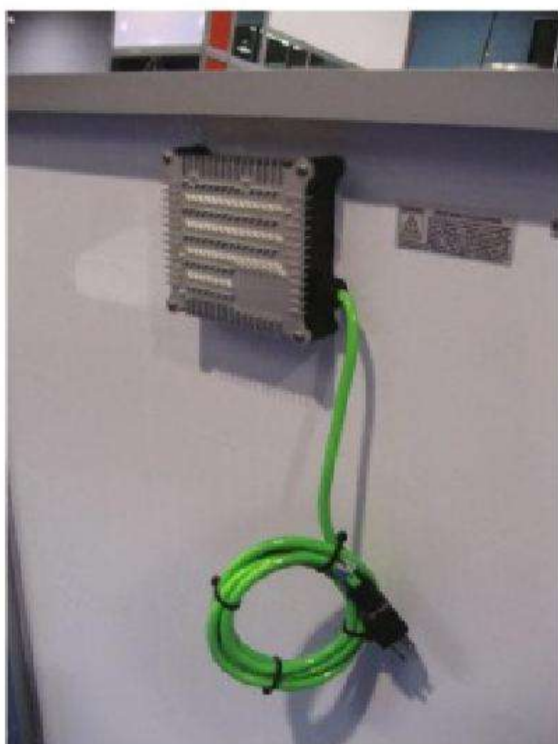
Figure 5.16 Micro-inverter attached to the back of a module
