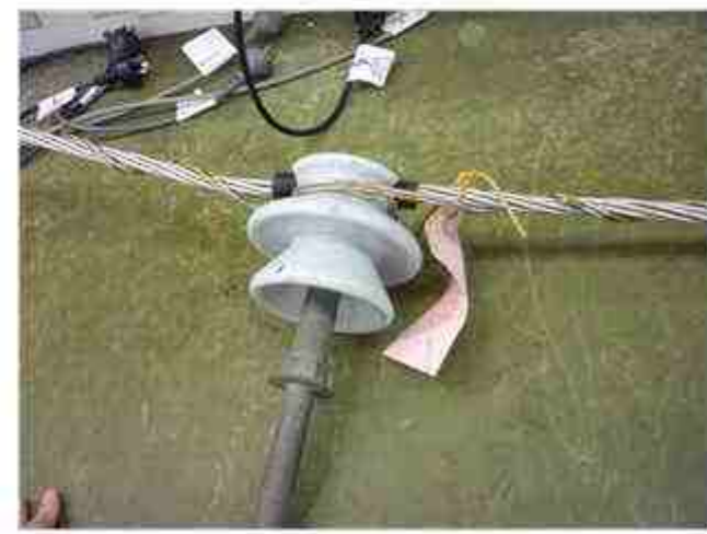
Page 285 Line insulator
