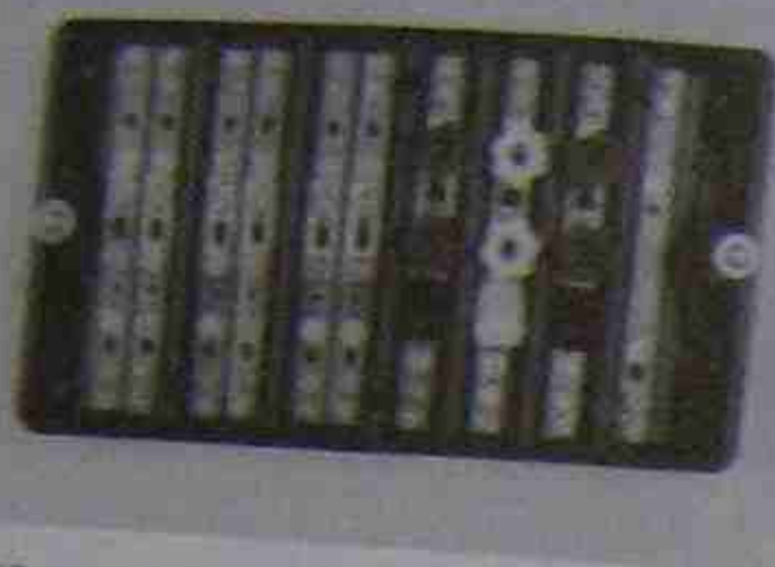
Figure 4.19: Example of a Meter Test Block
