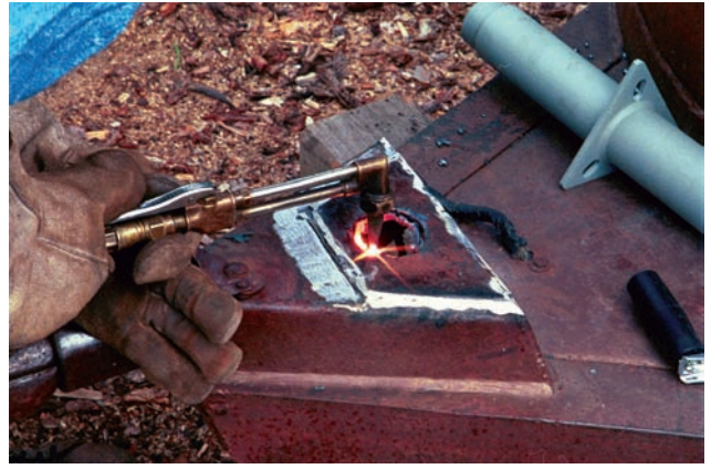
FIGURE 1-9 A hand cutting torch is being used to cut off the broken horse trailer jack so a new one can be welded in place. Courtesy of Larry Jeffus.
