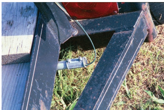
FIGURE 17-89(A) EMT protects trailer wiring. Courtesy of Larry Jeffus.
