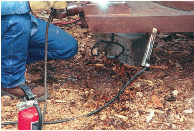
FIGURE 8-35 Make sure you have a good ground connection close to your welding. Courtesy of Larry Jeffus.
