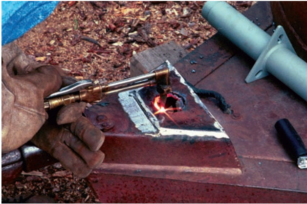
FIGURE 6-54 Bracing your hand on the tractor tongue will help keep you steady as you make the cut. Courtesy of Larry Jeffus.
