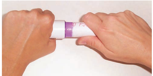
FIGURE 18-78 Insert the pipe into the fitting; then rotate 90 degrees and hold for 15 seconds. Courtesy of Larry Jeffus.
