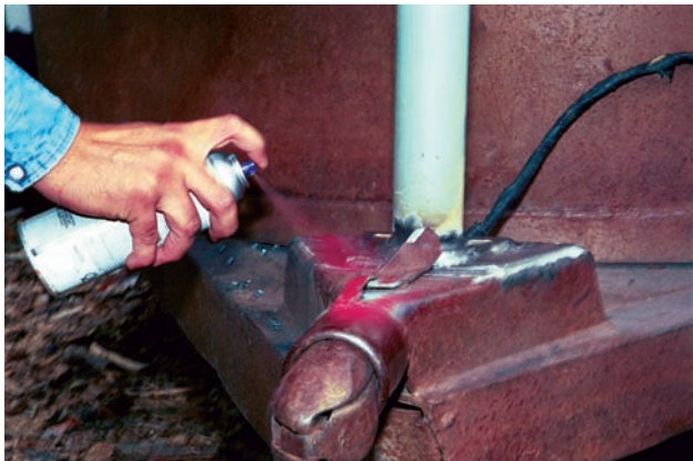
FIGURE 17-76 Spray paint the finished weld to keep it from rusting. Courtesy of Larry Jeffus.
