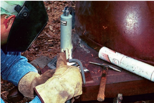
FIGURE 9-1 Stick welding is an excellent process to be used for most farm or ranch repair work. Courtesy of Larry Jeffus.
