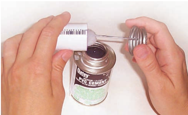
FIGURE 18-77 Apply PVC solvent to the inside of the coupling. Courtesy of Larry Jeffus.
