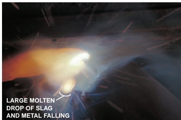
FIGURE 14-44 Hold the gun so that weld spatter will not fall onto the gun. Courtesy of Larry Jeffus.
