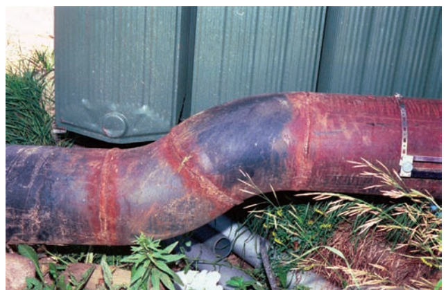
Welded irrigation pipe, Red River Ski Area.
