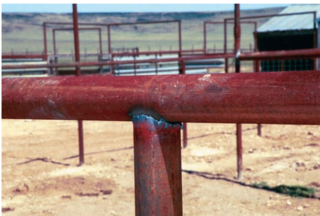
FIGURE 10-51 Pipe joint cut and fitted, ready for cleanup and welding. Photo courtesy of Larry Jeffus.
