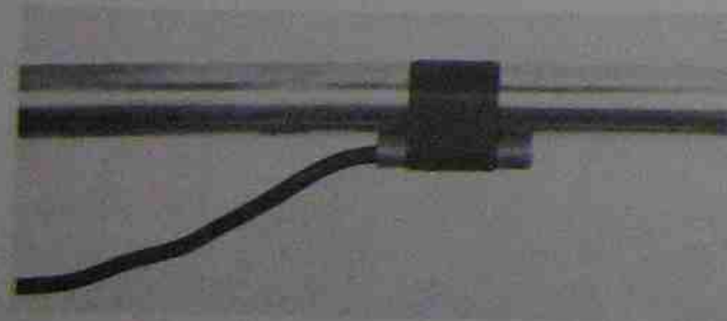
Figure 43-12. Temperature lead attached to a refrigerant line in the correct manner. It must also be insulated. Photo by Bill Johnson
