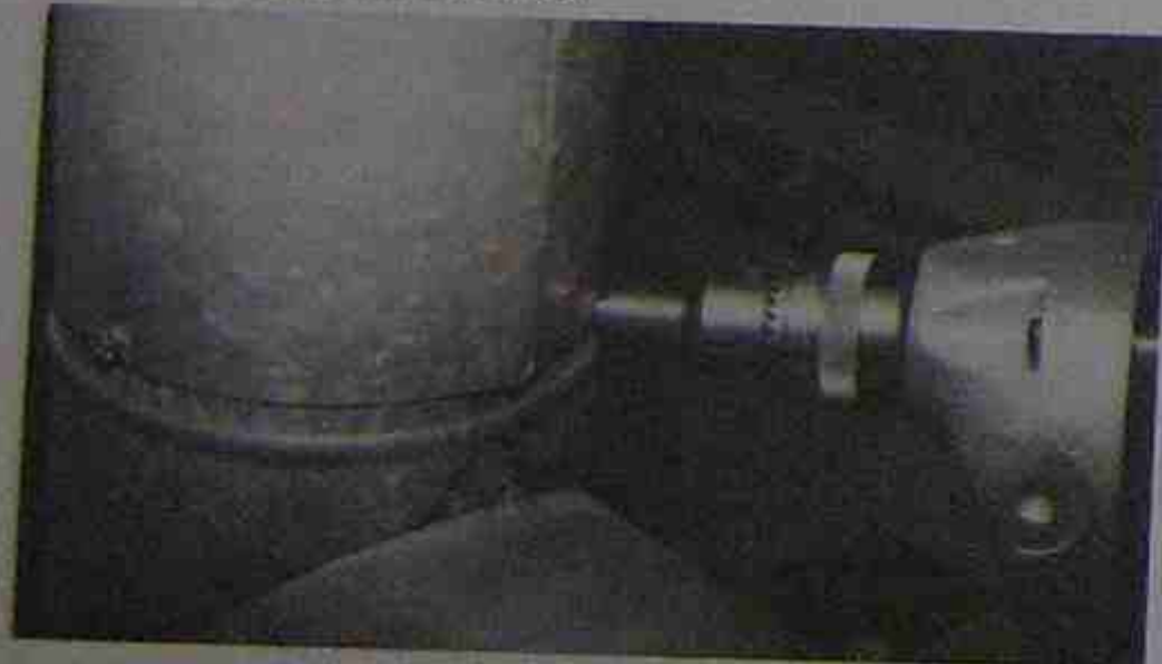
Figure 39-28. Fastening duct using a drill motor and sheet metal screws. Photo by Bill Johnson
