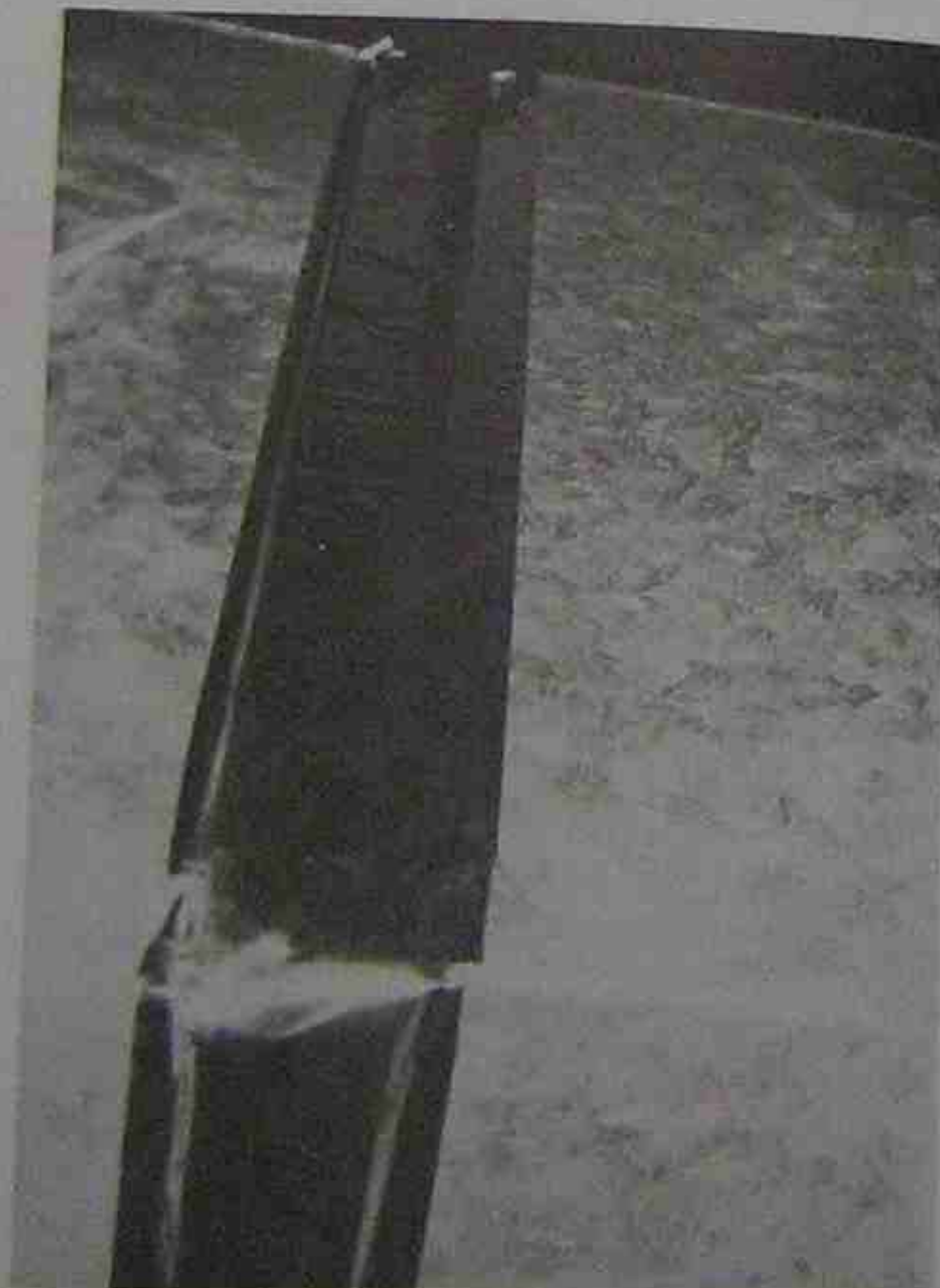
Figure 39-29. Taped duct connection. Photo by Bill Johnson
