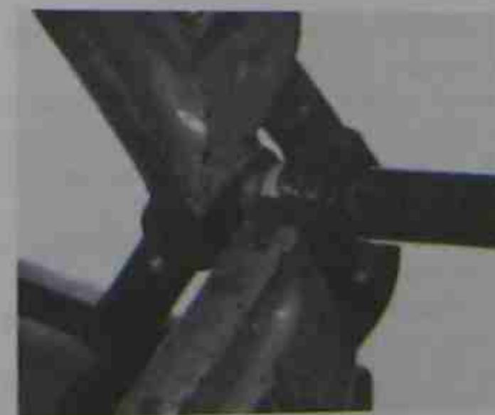
Figure 6-41. Holding pipe and turning fitting with pipe wrenches. Photo by Bill Johnson
