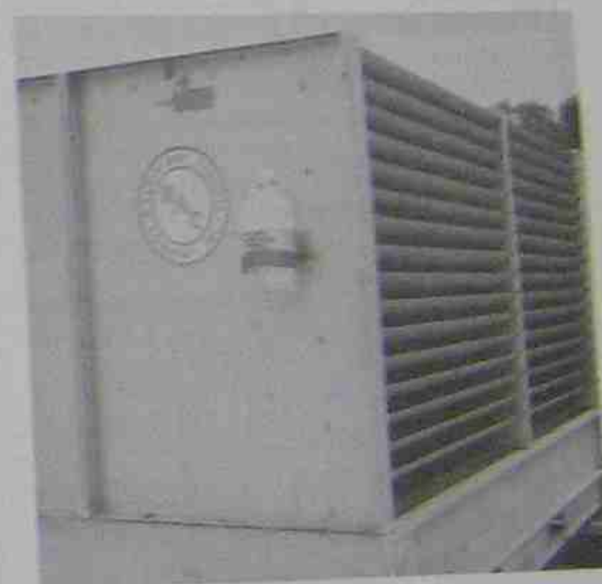
Figure 20-5. Method of adding water treatment to a cooling tower. Treatment is being metered at a rate that will last about a month so that the operator will not have to be in attendance at the tower all of the time. There is a constant bleed of the tower water to the drain to keep the water from being overconcentrated with minerals. Courtesy Calgon Corporation
