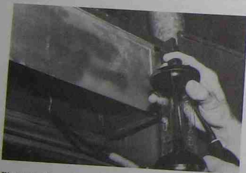
Figure 31-73. Sampling tube in draft diverter. Photo by Bill Johnson
