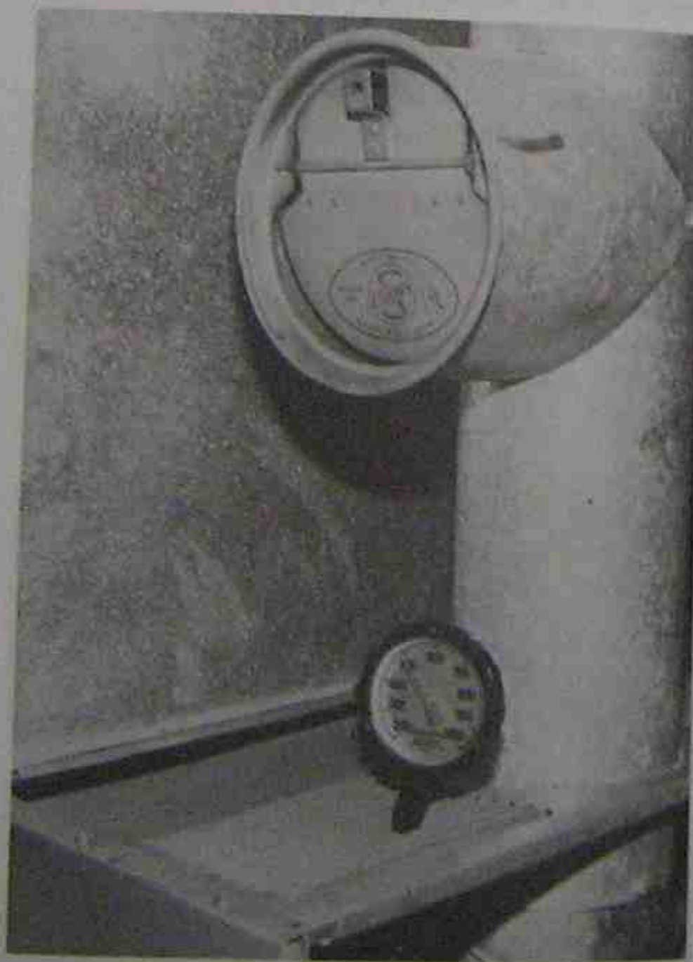
Figure 32-59. Making stack gas temperature test. Photo by Bill Johnson
