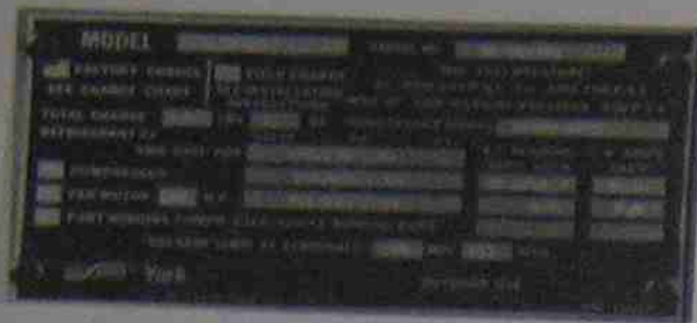
Figure 42-19. Condensing unit nameplate. Photo by Bill Johnson
