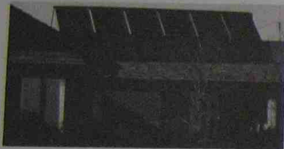
Figure 34-18. Typical collector installations.
