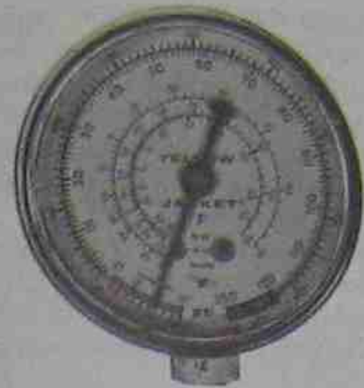
Figure 7-11. Manifold gage reading 20 in. Hg vacuum. Photo by Bill Johnson
