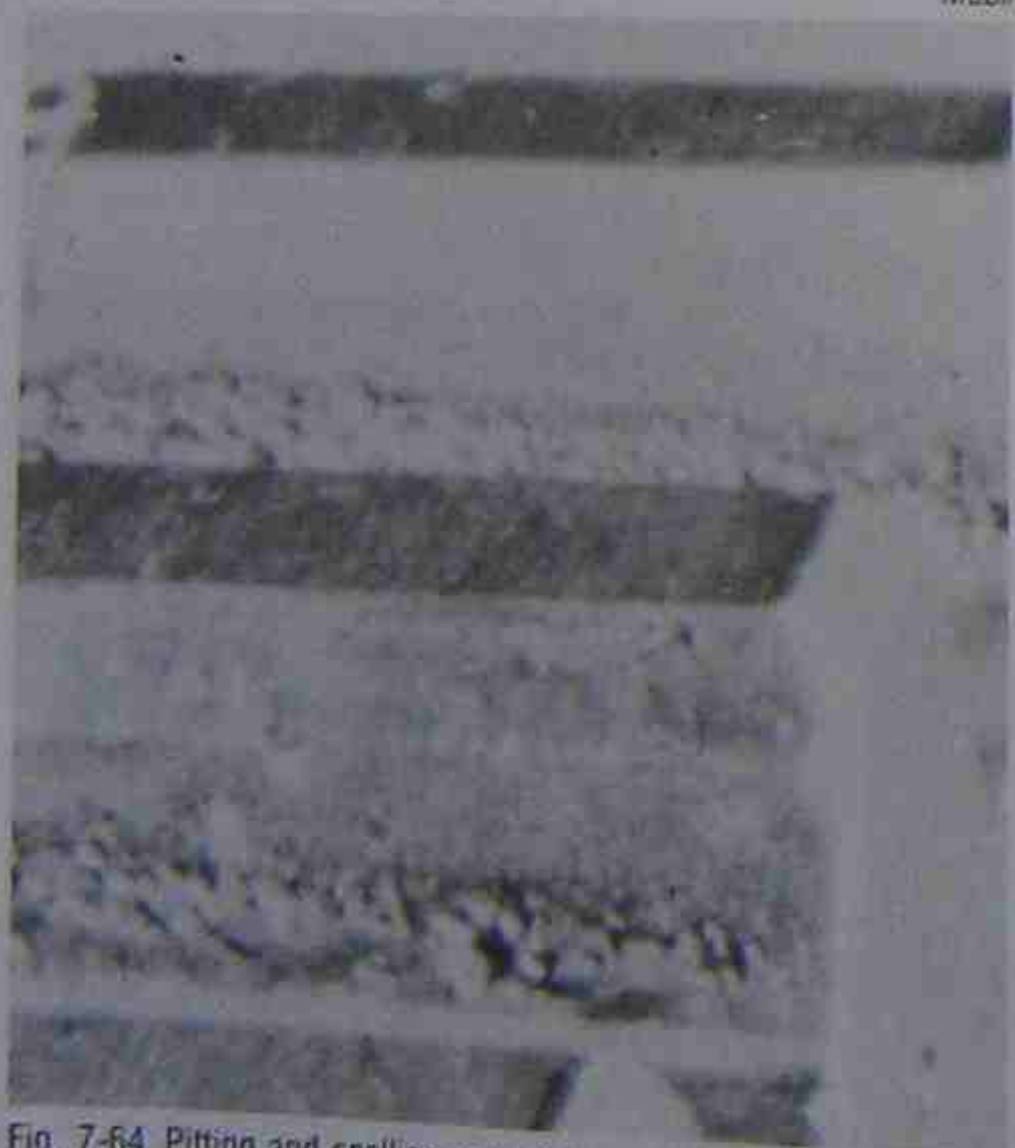
Fig. 7-64 Pitting and spalling caused by cyclical stress.
