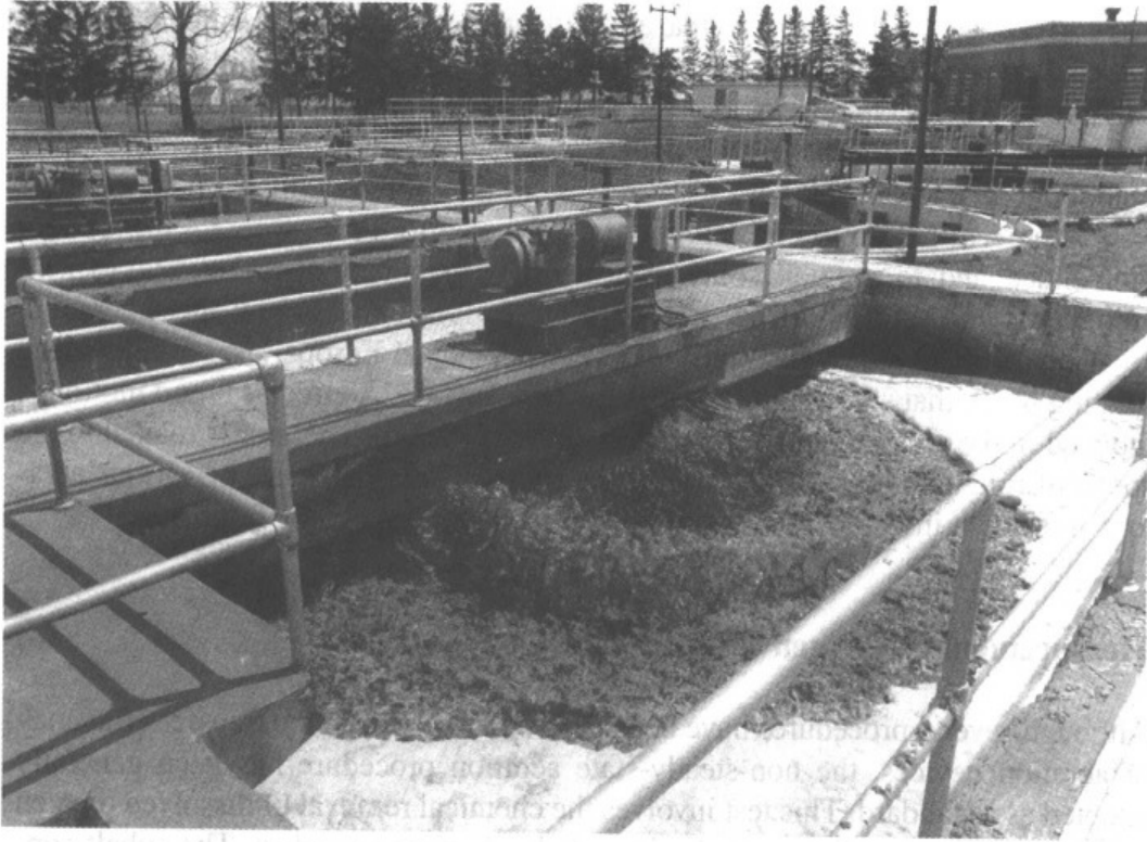
FIGURE 5.16 Low-speed surface aerator.
