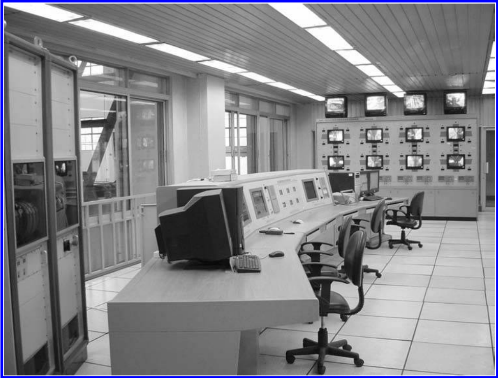
FIGURE 14.7 The control room.
