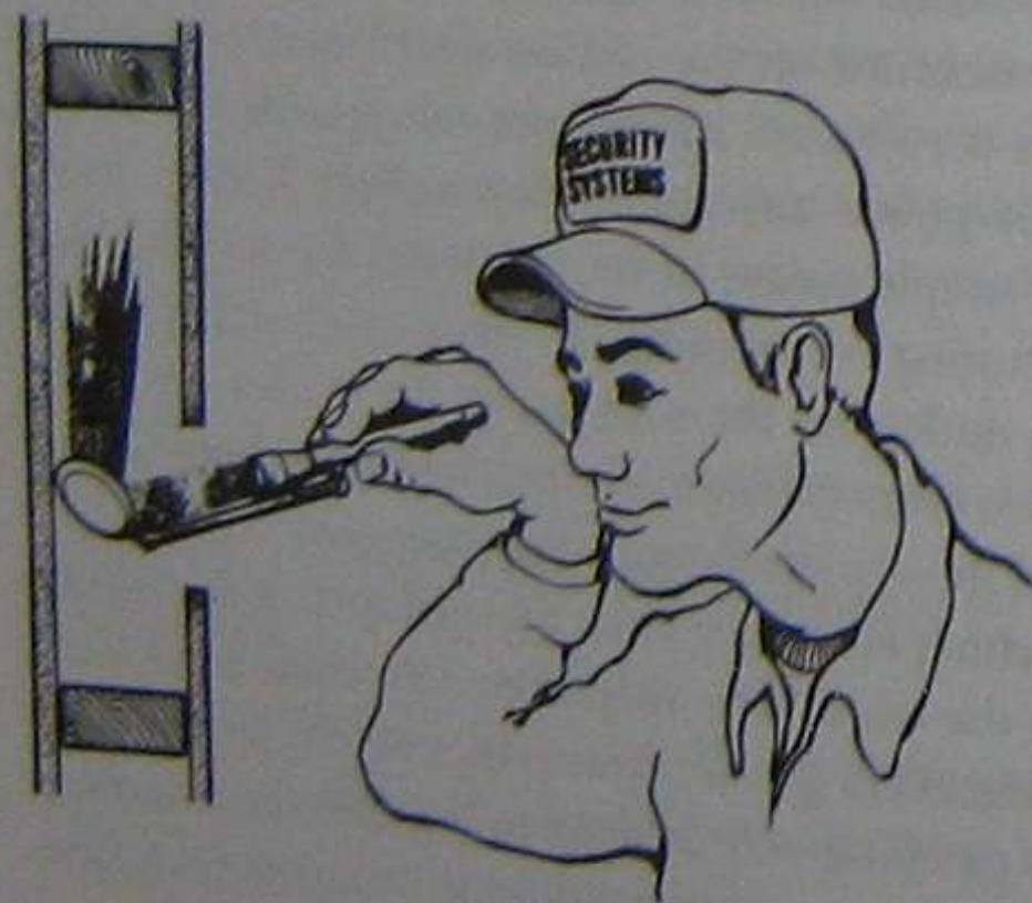
FIGURE 3-5. A flashlight and mirror used in combination are useful for viewing conditions inside of partitions.
