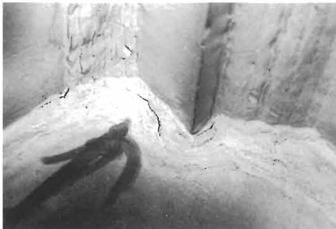
Fig. 4. Typical cracks found at external support welds.
