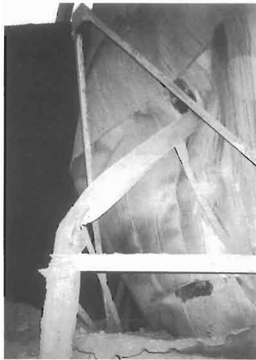
Fig. 3. View of buckled column.
