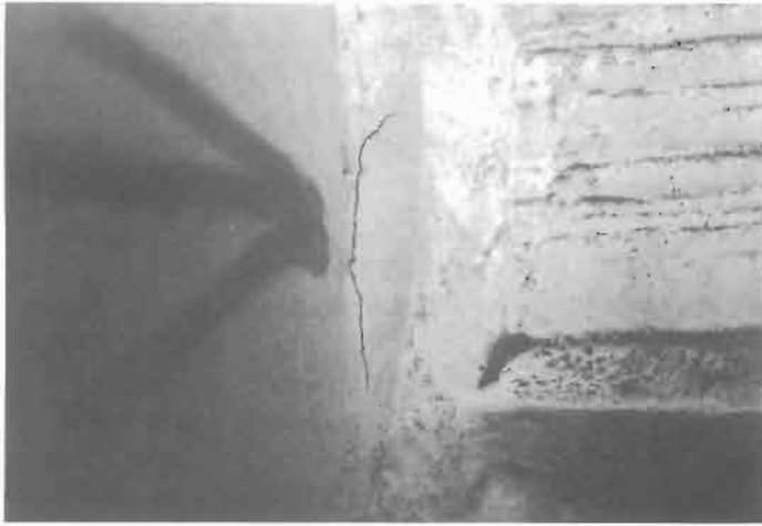
Fig. 5. Typical cracks found at external support welds.
