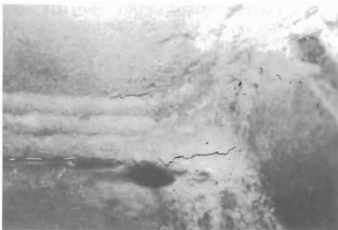
Fig. 6. Typical cracks found at external support welds.
