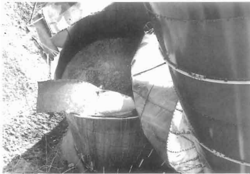
Fig. 5. Top view of failed silo, showing remaining filling level.
