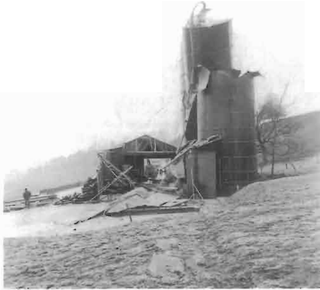
Fig. 1. Damaged silos: view of the site.
