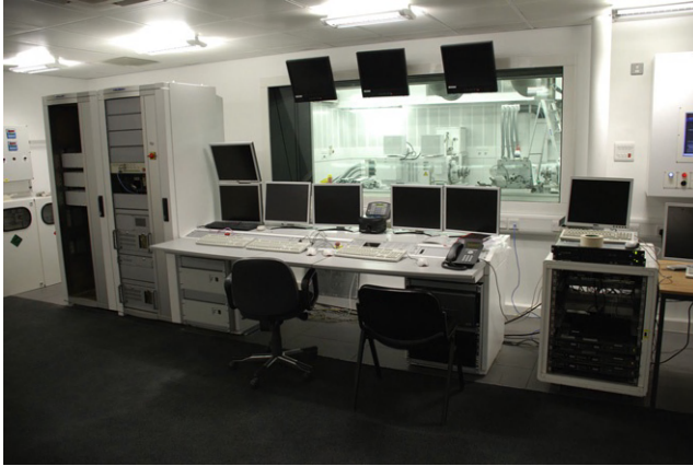
FIGURE 4.10 A general view of a modern powertrain test cell control room. Note that the screens above the cell window are dedicated to CCTV cameras inside the cell. The window is triple glazed. (Photo courtesy of Mercedes GP Petronas Formula 1 Team.)
