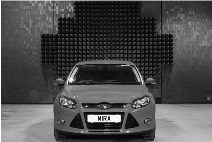
FIGURE 18.5 The mixed, pyramidal, and ferrite tile absorption lining on the end-wall of a large automotive EMC semi-anechoic test cell. Chamber dimensions: 20 m × 11 m × 7 m high. (Photo courtesy of MIRA Ltd.)
