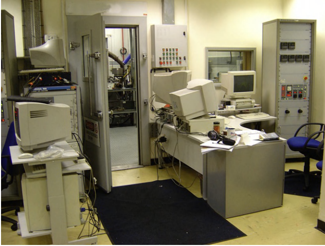
FIGURE 4.9 Part of a control room area that has a number of shortcomings arising from poorly integrated and ad hoc development.
