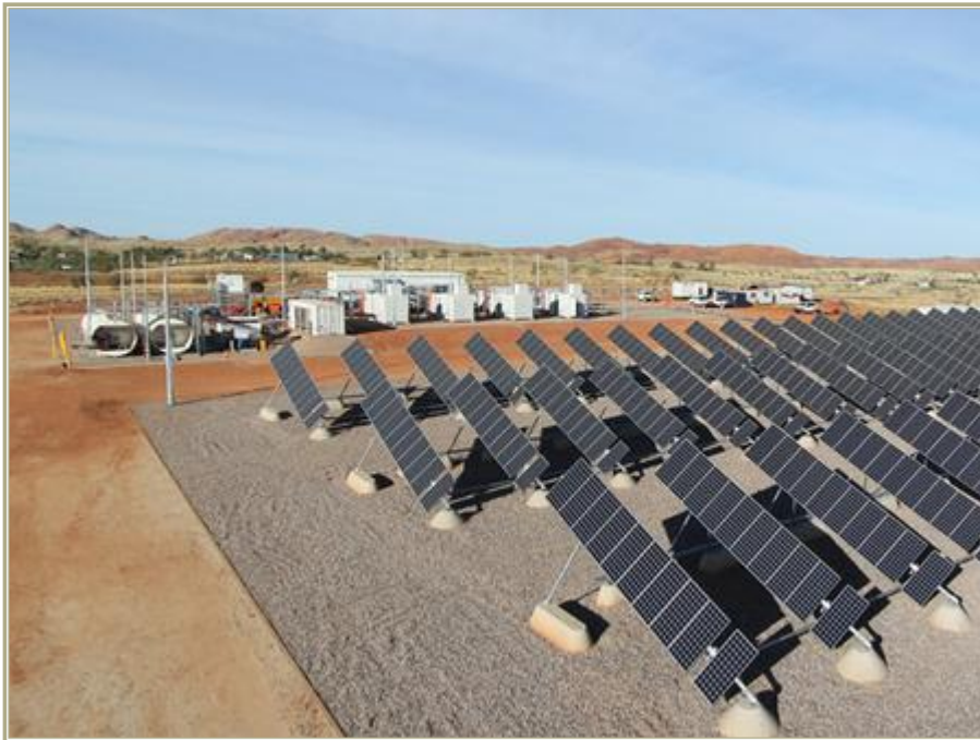
Figure 14: Marble Bar Power Station
