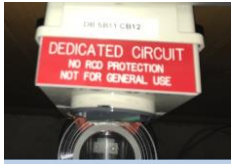
Figure 6 Dedicated circuit - example of required signage for GPO with RCD removed.
