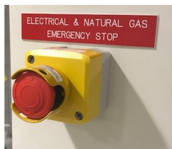
Figure 1 Example of electrical emergency stop red button.
