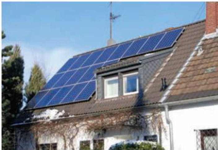
1500 W domestic solar panel installation
