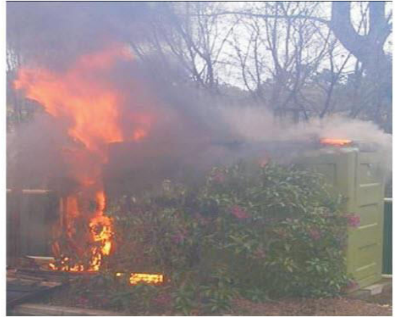
Pad mount transformer on fire
