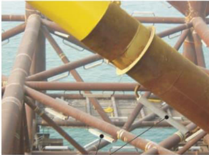
sacrificial zinc anodes on a steel structure
