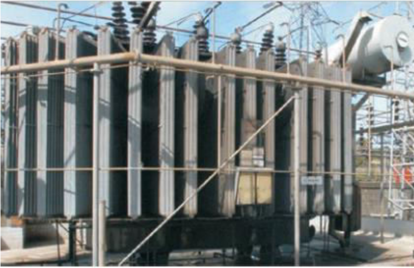
power distribution transformer in a substation
