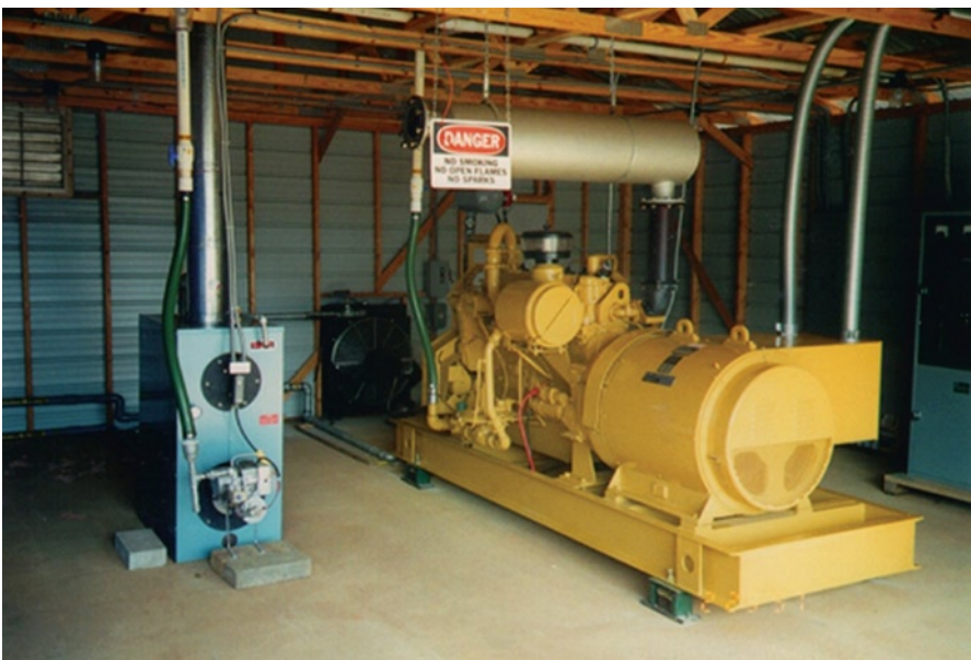
Fig. 2.8 Generator set utilizes biogas, for generating electricity (photo courtesy: AgSTAR)
