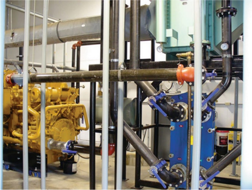
Fig. 2.9 A heat exchanger working with a biogas-fed engine-generator set to utilize heat for space and water heating (photo courtesy: AgSTAR)
