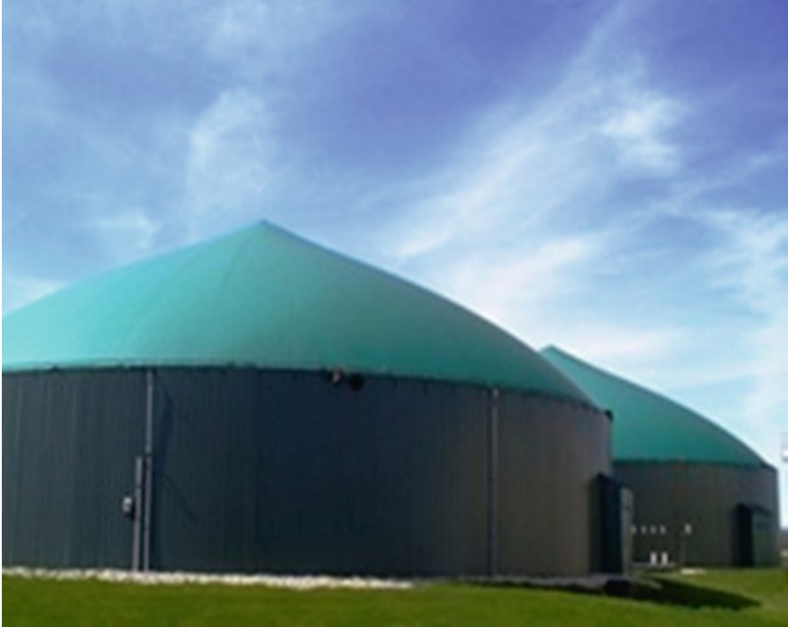
Fig. 5.14 Completely mixed digester (Photo courtesy: AgSTAR)
