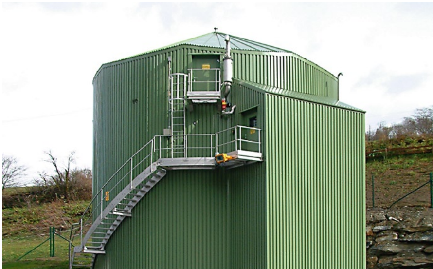
Fig. 7.10 A BIMA digester processing 11,000 tonnes per year of municipal sewage sludge at Tamsweg, Austria (photo courtesy: Entec biogas)
