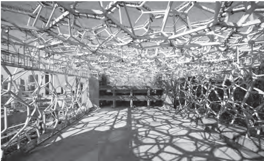
FIGURE 9-4-9 Interior view of the Water Cube pavilion showing the steel structure nearing completion. Image courtesy Ben McMillan and Arup.
