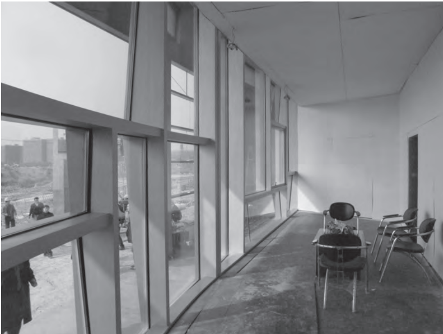
FIGURE 9-6-5 Photo of a 15 ft. × 42 ft. visual mock-up, fabricated by SGT in Shenzhen, China.
