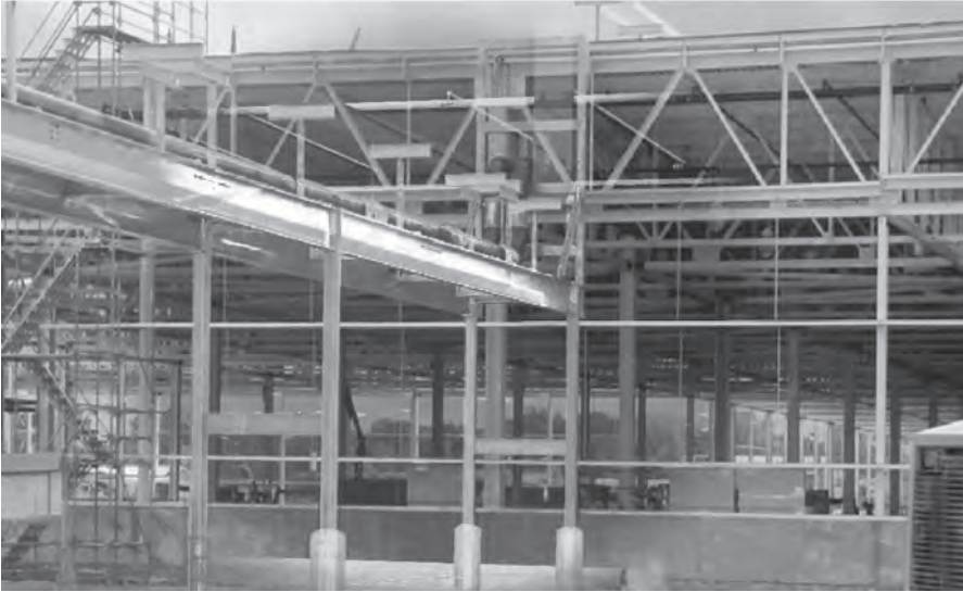
FIGURE 9-1-7 Overlay of the model with the built project demonstrates the 'as-built' nature of the model.
