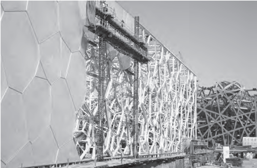
FIGURE 9-4-8 Construction of the Water Cube pavilion. Image courtesy of Ben McMillan and Arup.
