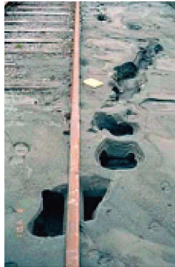
Sand ejected through a crack forming a series of sand boils along the railroad tracks adjacent to Deschutes Parkway in Olympia. (Photo courtesy of geomatrix)
