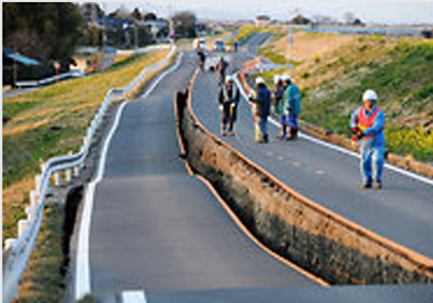
Figure 6.4 Damage to a road in Saitte, in Saitama Prefecture, from the Kobe earthquake.
