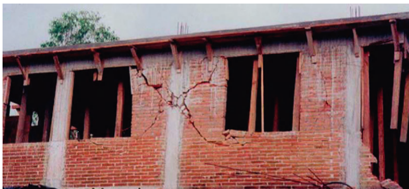
Figure 11.1 Earthquake damage of a confined masonry building during 1999 Tehuacan earthquake (as reported by EERI, 1999).
