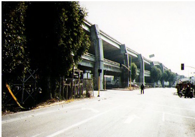
Figure 4.5 Northridge earthquake damage.
